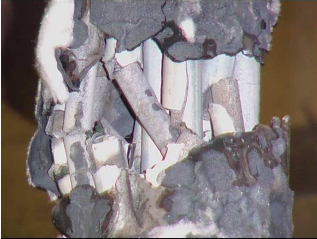
Figure 3.22 Detail of heater rod rubble
