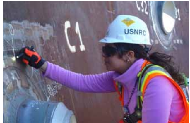
Division of Engineering (DE) General Engineer Marieliz Vera inspects the weld of a Vogtle Unit 4 containment penetration.
