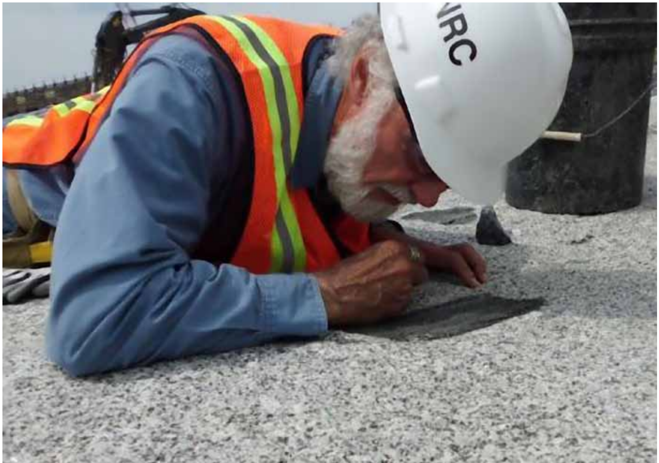
At the V.C. Summer Unit 3 site, NRC Senior Geologist Gerry Stirewalt takes an “up close and personal” look at the foundation grade level bedrock surface.
