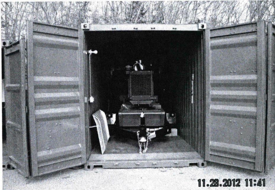
Typical Godwin Pump storage, with power for block heaters and battery charging.
