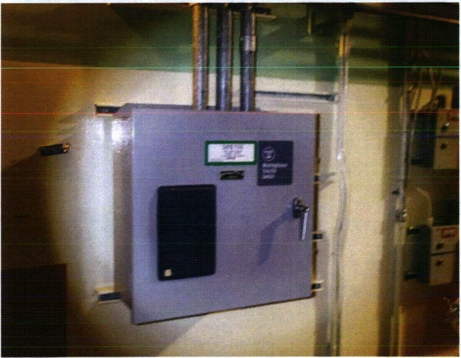
Equipment ID: 30S703
