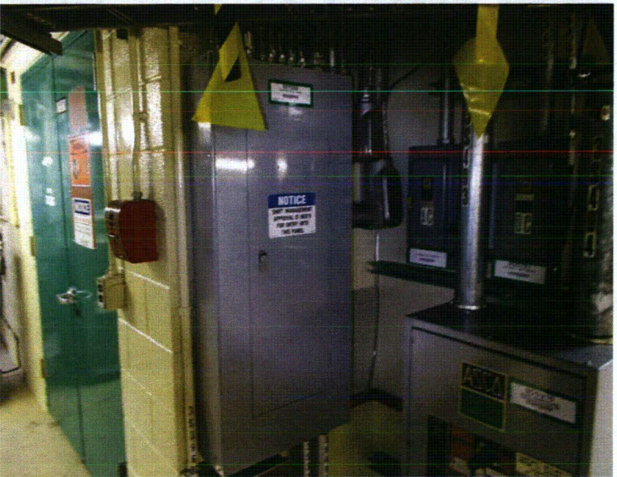
Equipment ID: 30Y050
