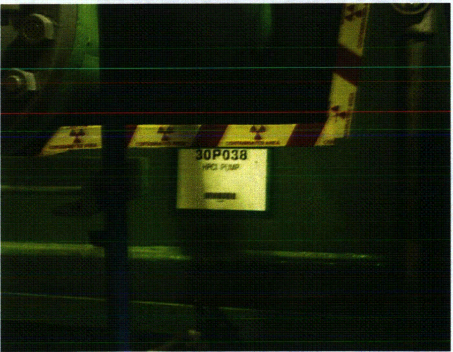
Equipment ID: 30S037
