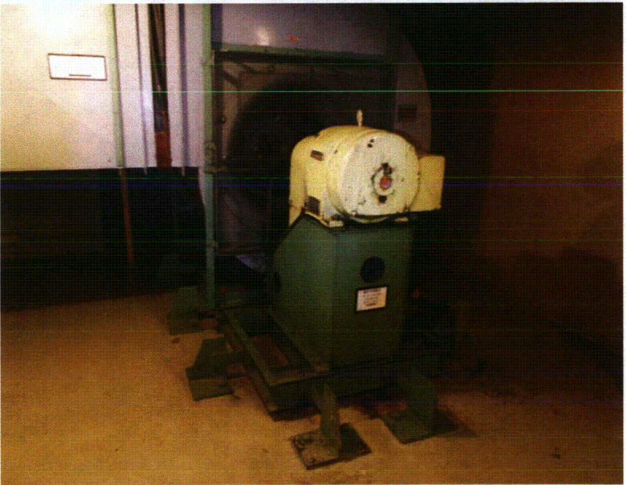
Equipment ID: ODV064
