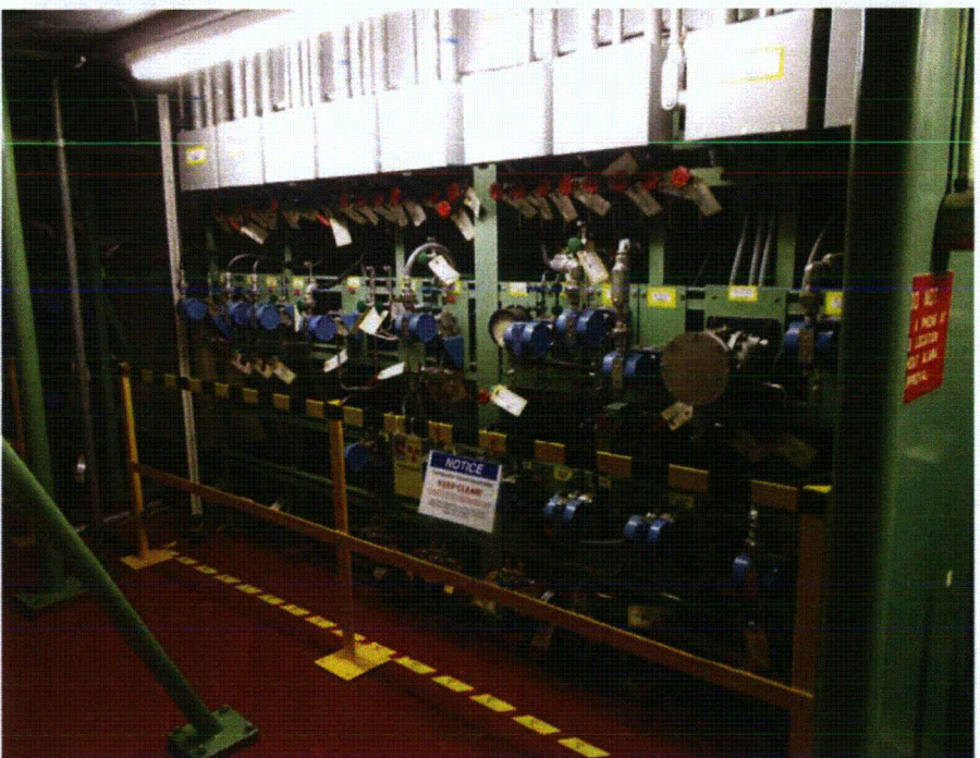
Equipment ID: 2AC065
