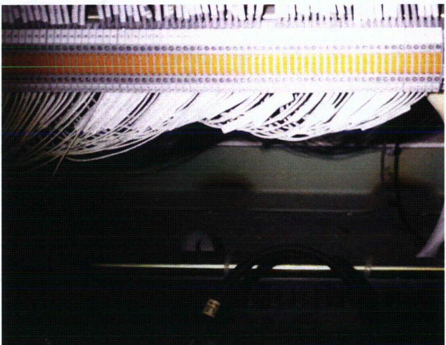
Equipment ID: 20C006C
