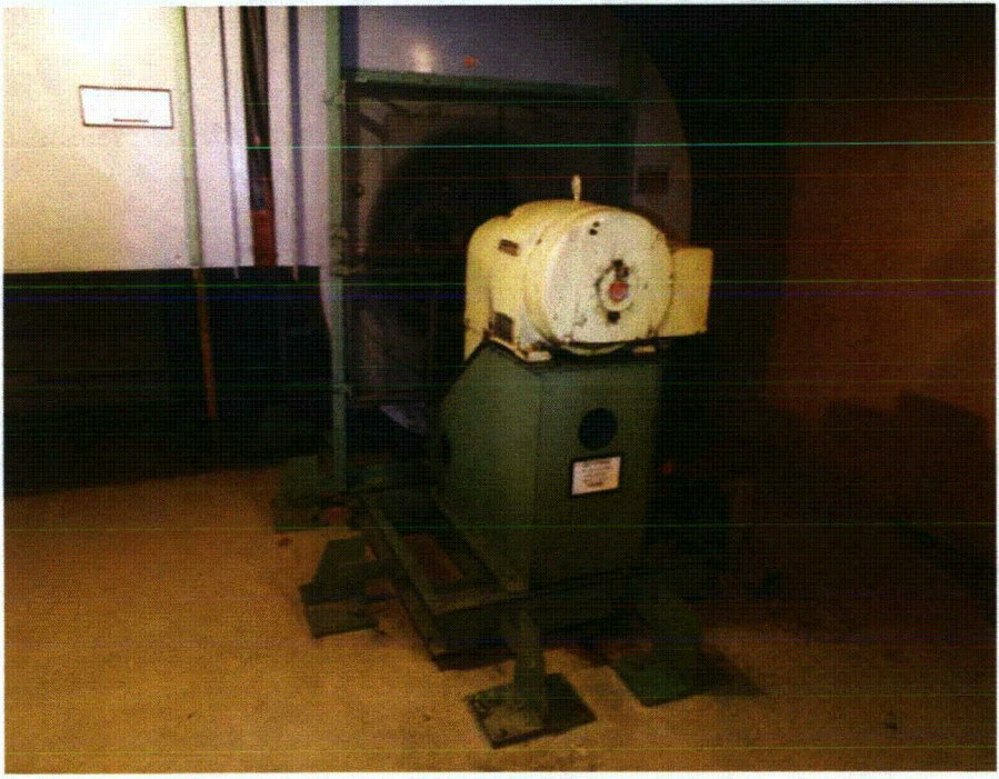
Equipment ID: ODV064
