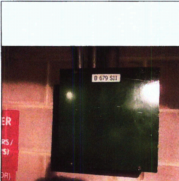
Note: Left side (top and bottom) screws are missing. Junction box is about 3' from the valve
