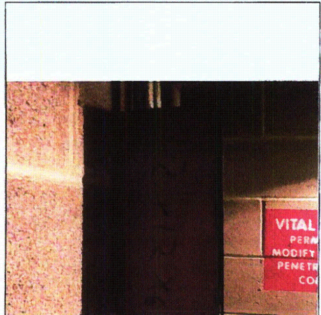
Note: Left side view of # B 679 SII showing gap resulting from missing screws.
