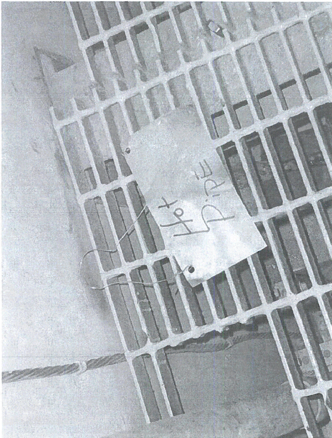
Figure 2 – Hot Pipe Sign (Unit 2 HPCI Room)
