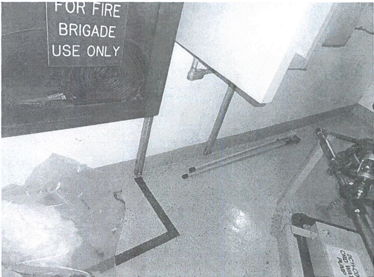
Figure 3 Poles/Handles Stored on Floor Near Hose Station
