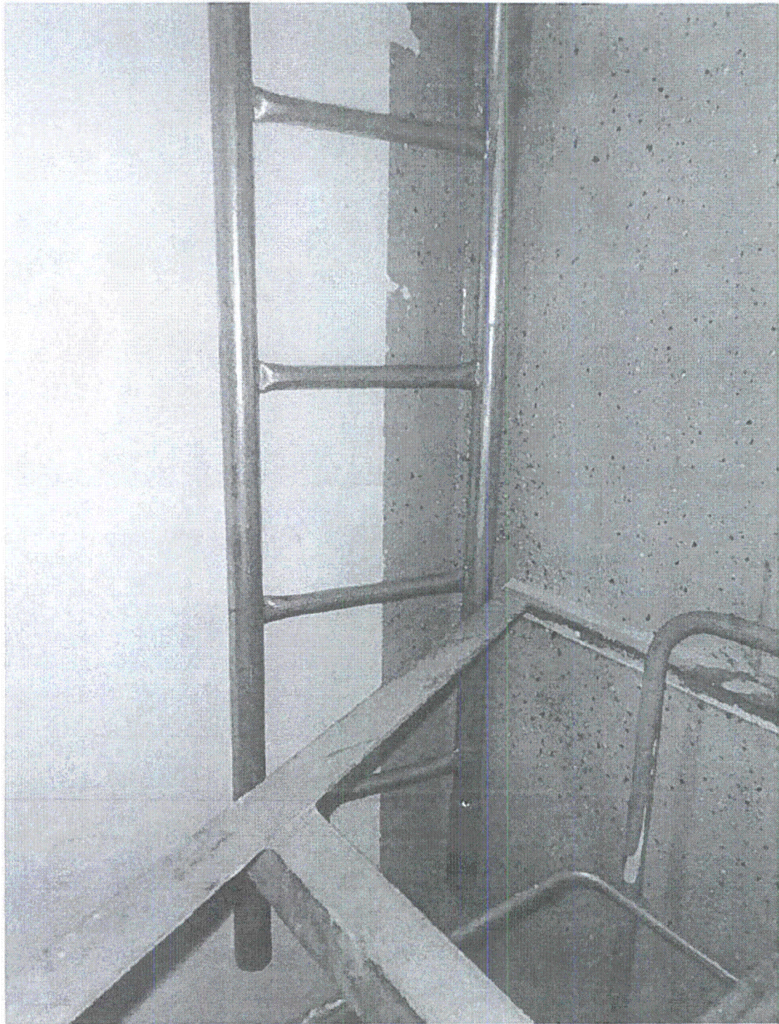
Figure 4 – Unrestrained Metal Ladder (Unit 2 87' NE Diagonal)
