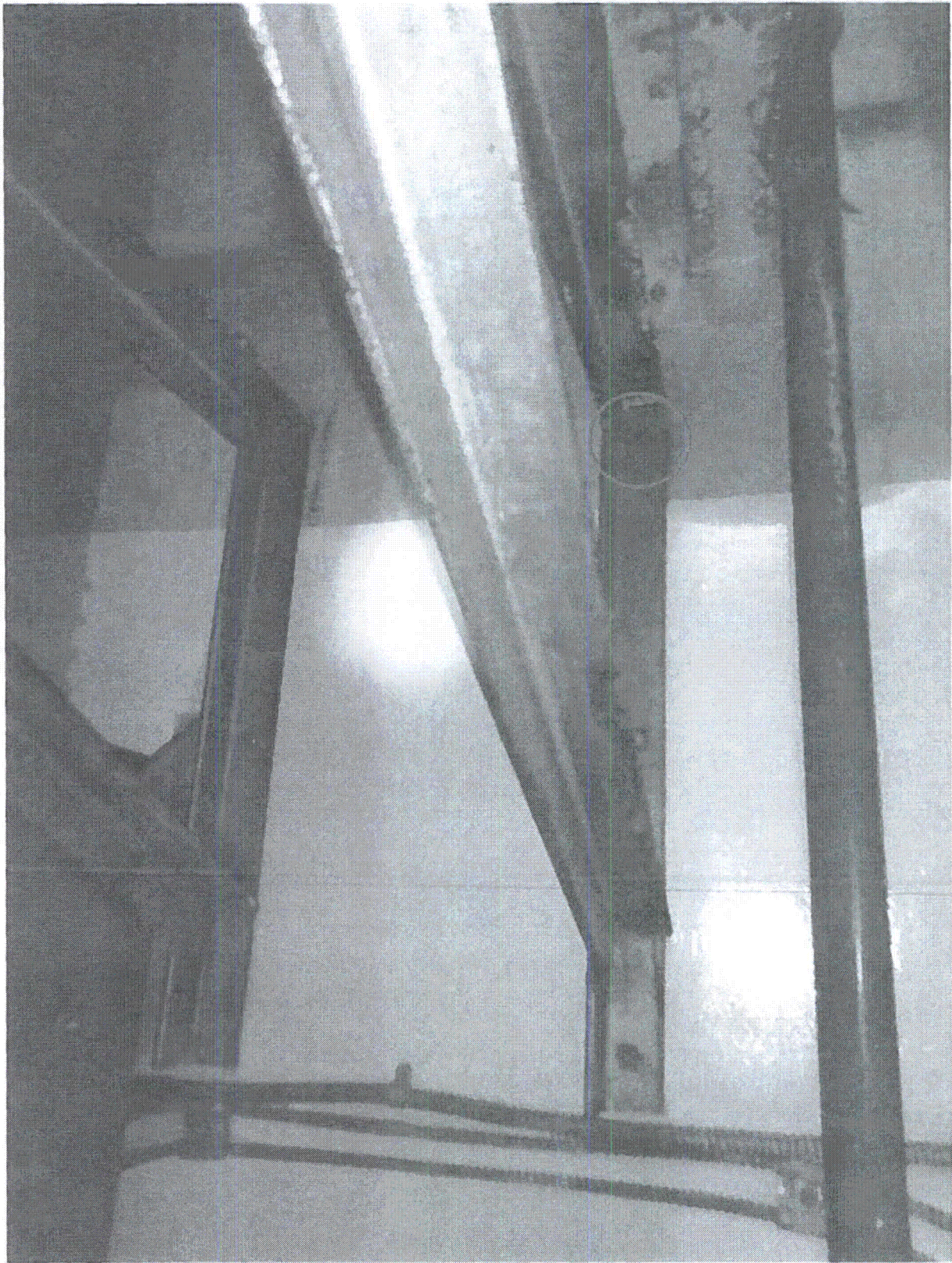
2: Missing Anchor for Cantilever Support Off West Wall (2R103)
