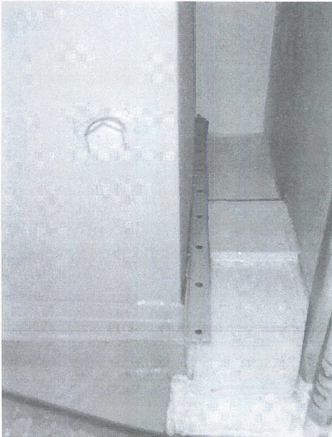
Figure 2 – Missing HVAC Bolts (Room C-114)
