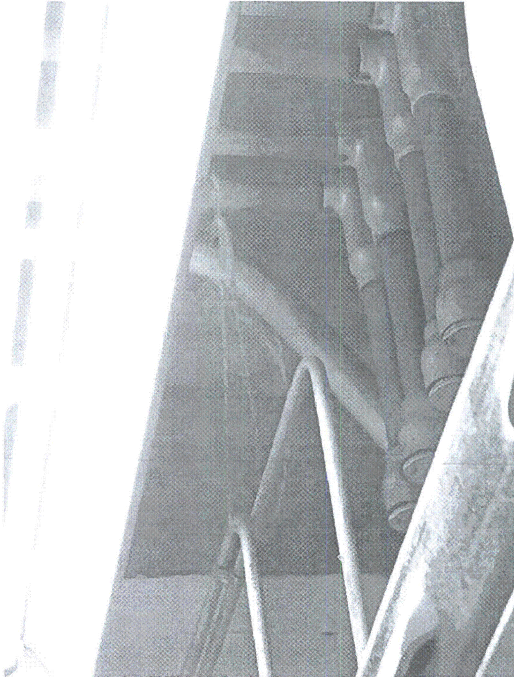
Figure 1 – Instrument Tubing Tied to Conduit (C140)
