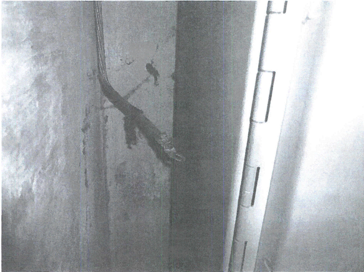
1: Unattached Ground Cable to 2H21-P293 (Battery Room 2C)
