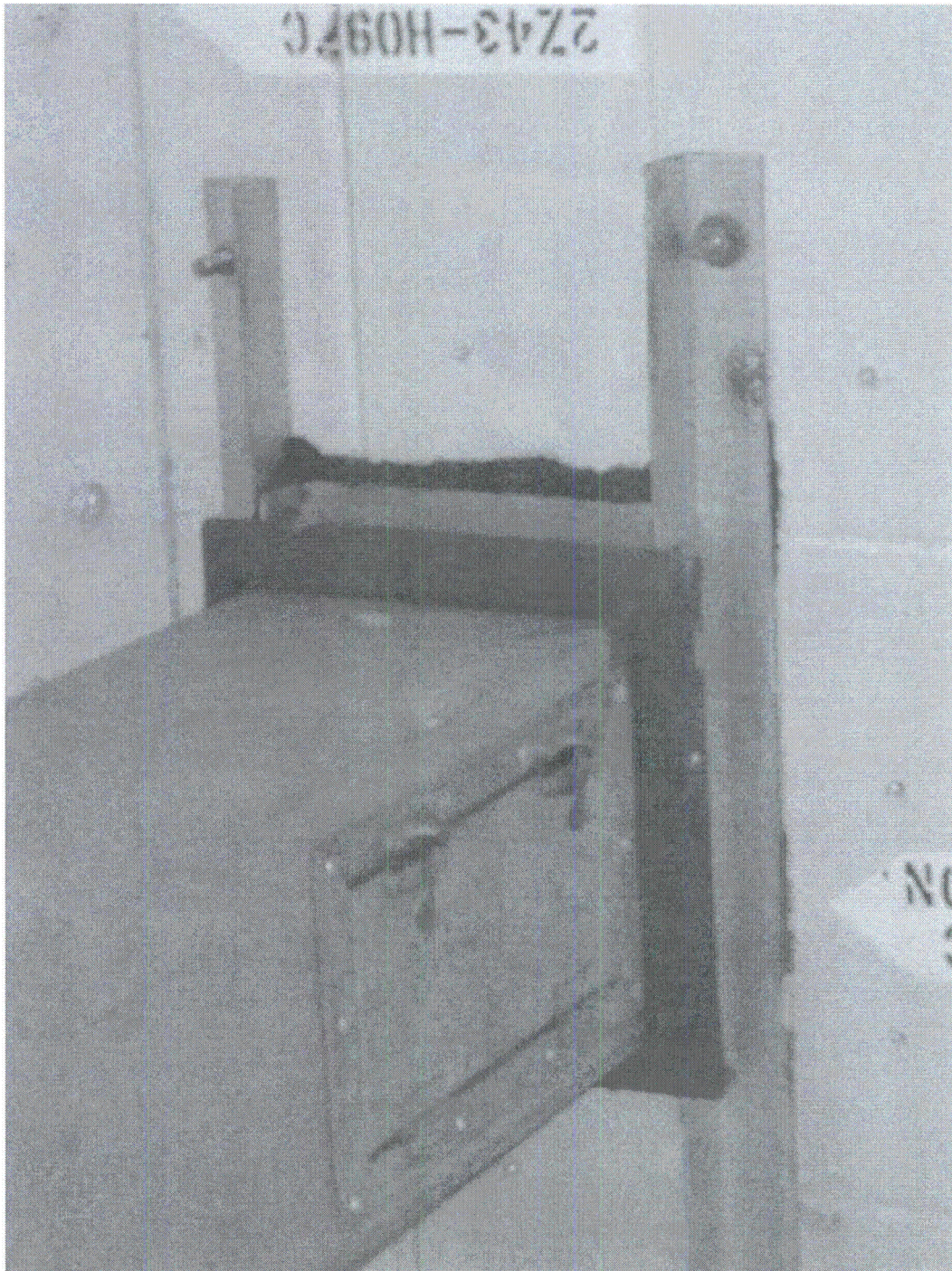
Figure 1 – Difficult to See Nut on Anchor Bolt (Room C-027)
