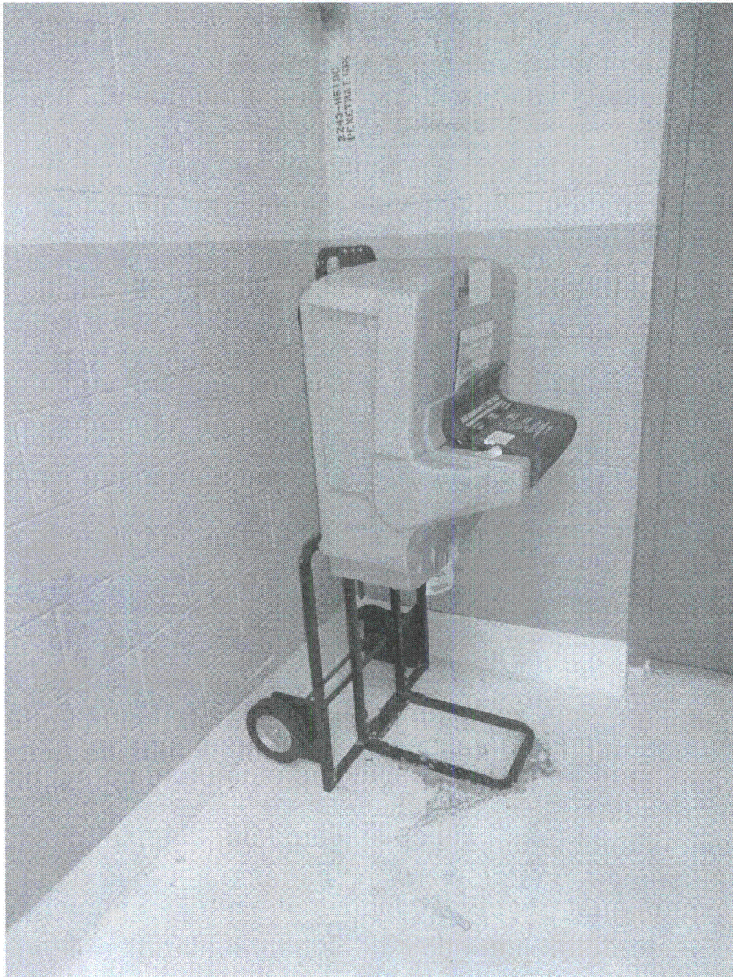
Figure 2 – Broken Eyewash Station (TC-T12 Control 112)
