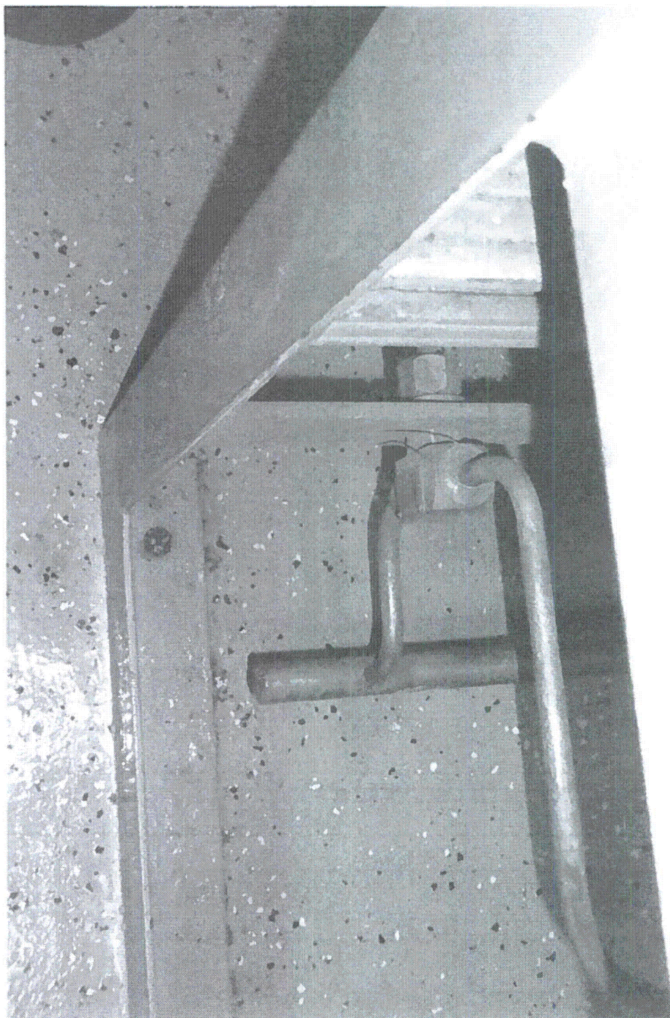
Figure 3 – Missing Anchor on Rack Support (2H21-P021)
