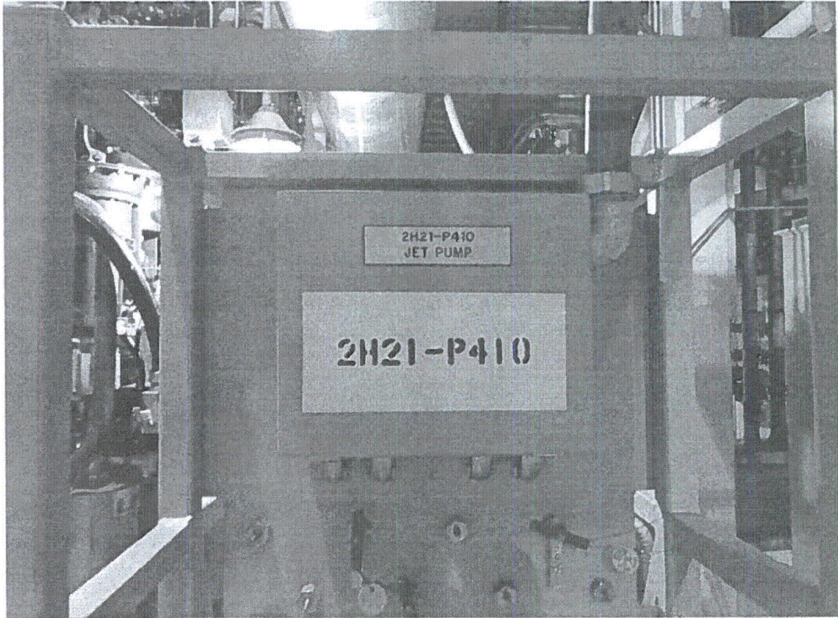
Figure 1 Equipment ID (2H21-P410)
