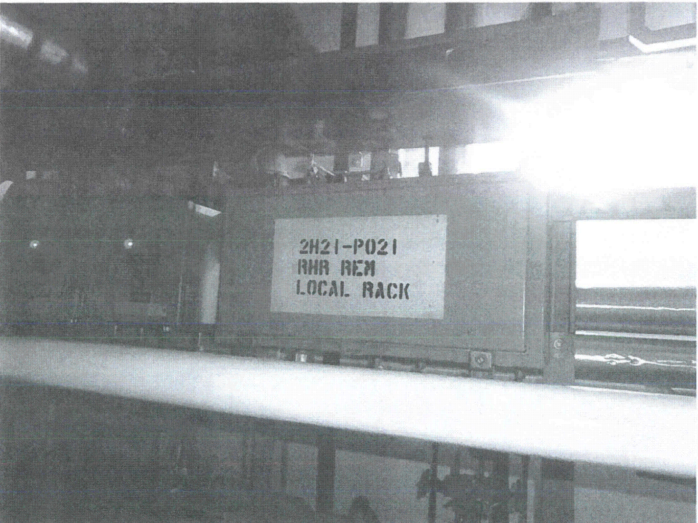
Figure 1 – Equipment ID No (2H21-P021)
