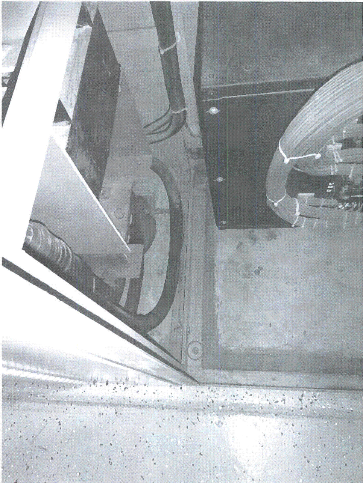
3: Missing Plug Welds (2R43-P001C)
