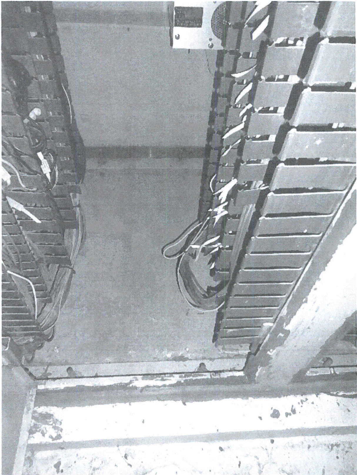
3: Loose Cables Inside Cabinet (2C82-P001)
