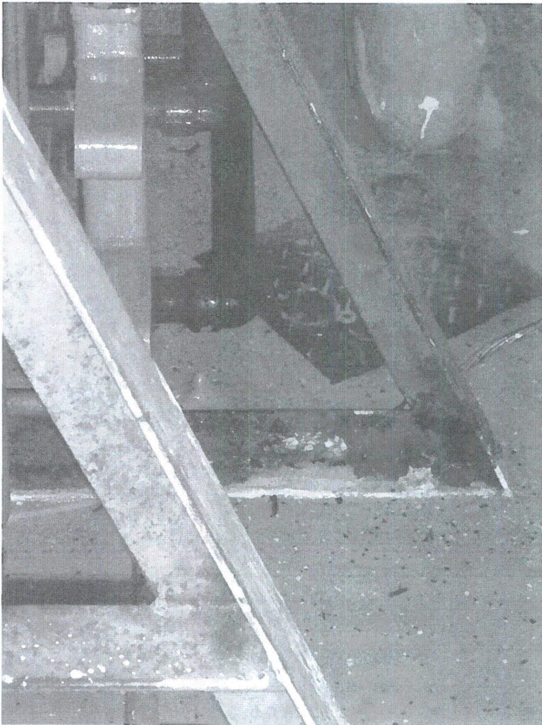
Figure 3 – Mild Oxidation on Anchor Bolts (2H21-P018)
