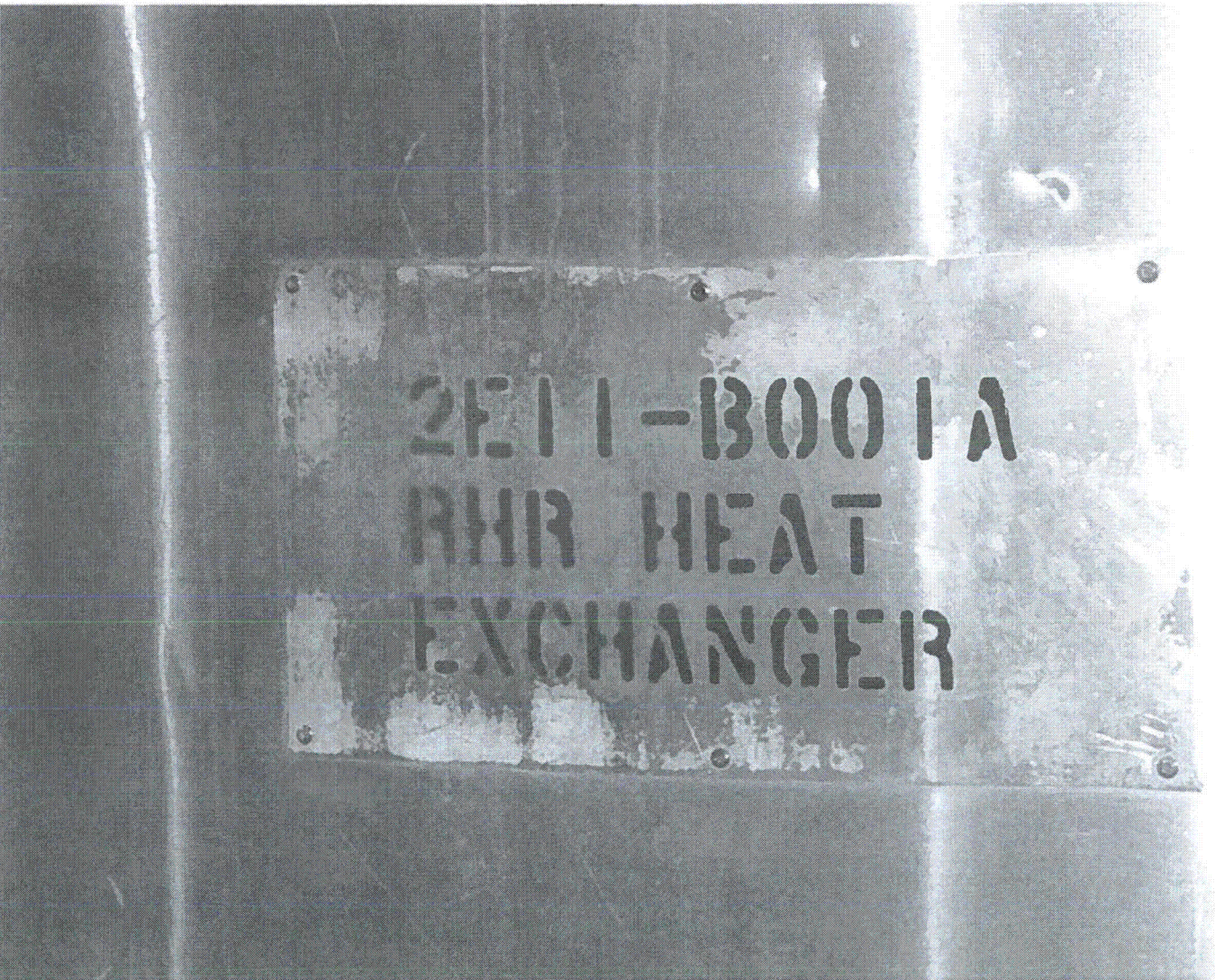
Figure 1 – Equipment ID No (2E11-B001A)
