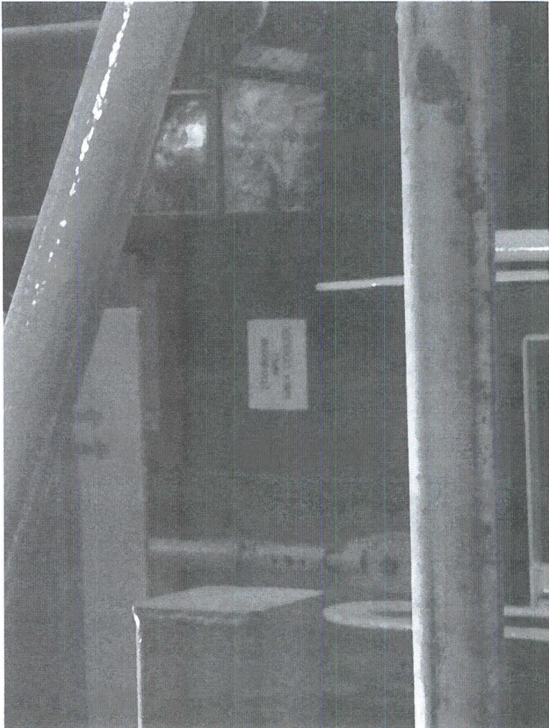
Figure 1 – Equipment ID No (2T41-B005B)
