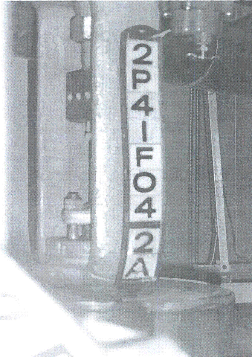
Figure 1 Equipment ID: 2P41-F042A
