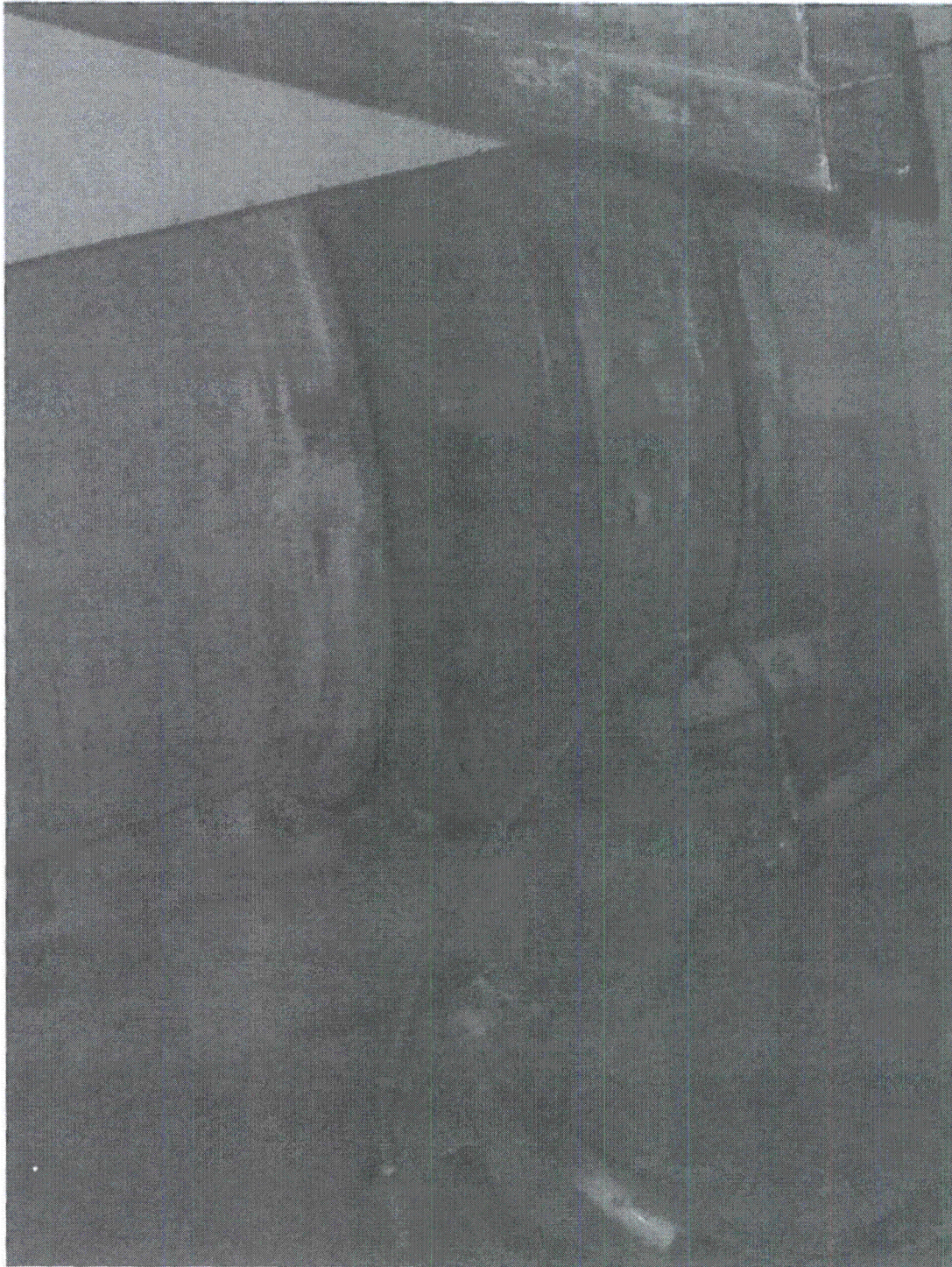
Figure 3 -- Mild Oxidation on Flange Bolts (2T41-F004A)
