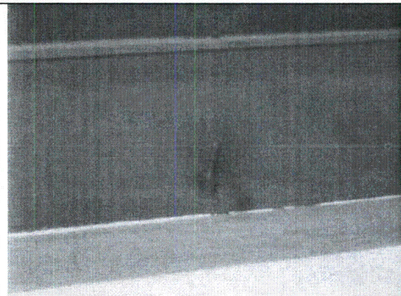
Note: Anchor bolt slightly tilted
