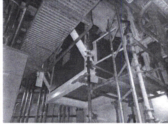
Note: General view of the cooler
