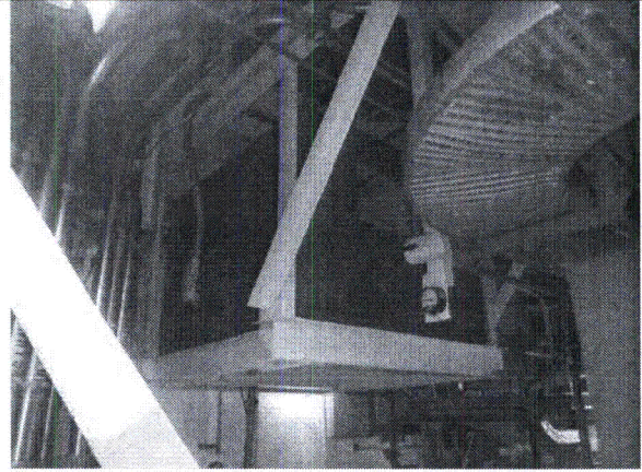
Note: General view of the cooler
