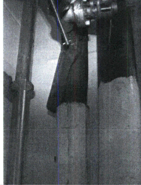
Note: Surface oxidation on pipe
