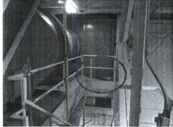
Note: Controls for the overhead hoist.
