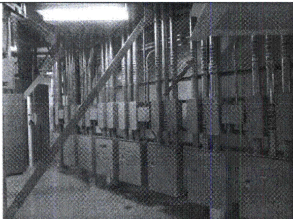
Note: Conduits from cable tray
