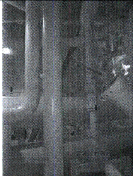
Note: Ladder in the area
