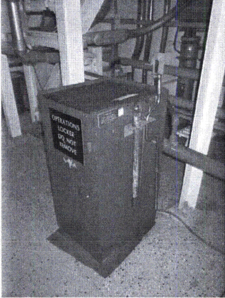
Note: Operations Locker on floor
