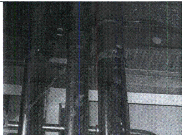
Note: Only conduit without unistrut support clamp at this location
