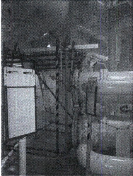
Note: Ladder in the area
