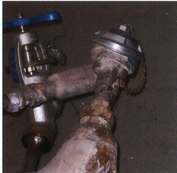
Note: Temperature element closeup.
