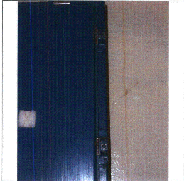
Note: Missing latches.
