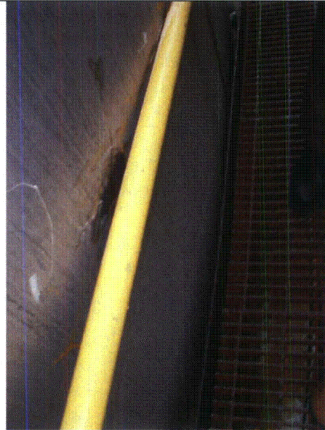
Note: The tank too close to the platform railing
