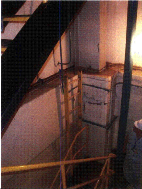
Note: Unsecured ladder next to stair way.
