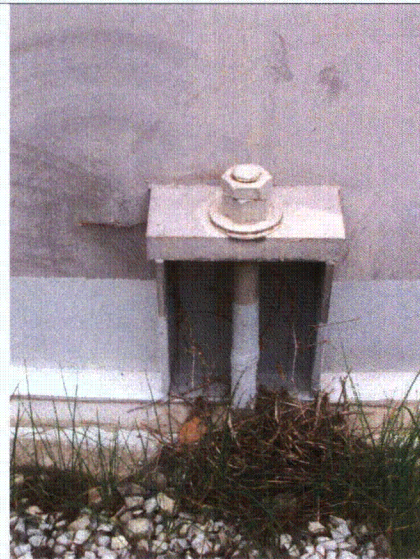
Note: Anchorage of the storage tank
