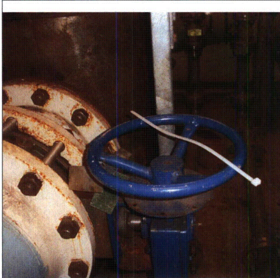
Note: Wire ties found lying loose in area.
