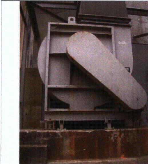
Note: 21 Electrical Tunnel Exhaust Fan
