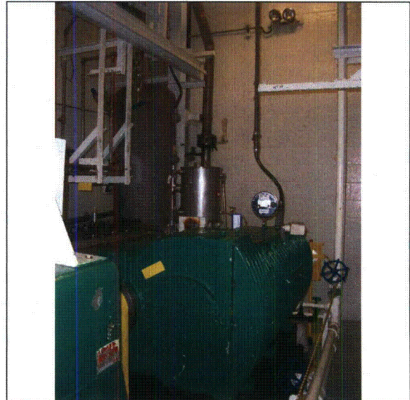
Note: 23 Charging pump room looking south.
