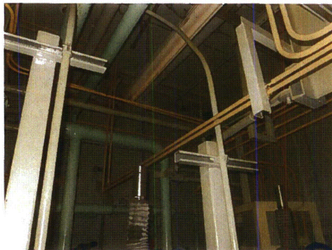
Tubing with excessive distance between supports at entry to room.
