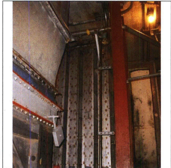
Note: HEPA filters behind fan 22.
