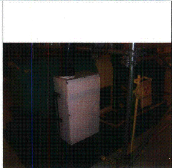
Note: View of pump
