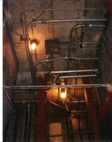
Note: Overhead area with 22 fan on left.
