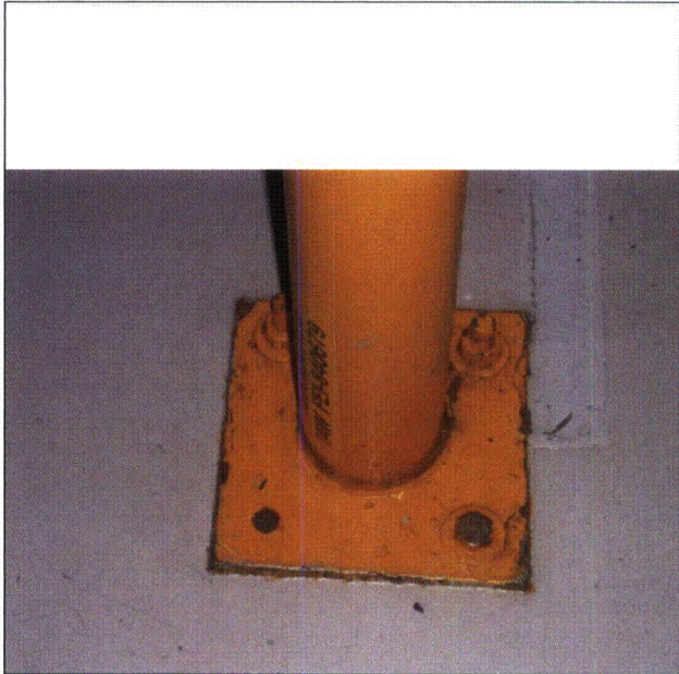
Note: Trolley stanchion with missing anchor bolt.
