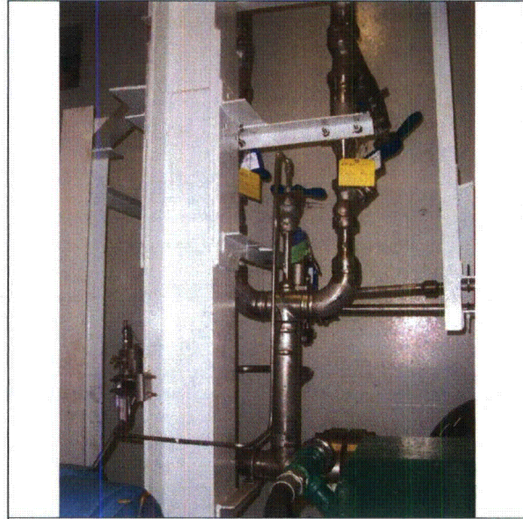
Note: Pipes coming off of the 23 charging pump.
