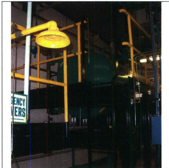
Note: Ladder safety chain kept unattached on Component Cooling Surge Tank platform ladder. CR IP2-2012-06354 issued to track resolution.
