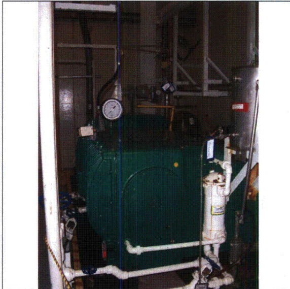
Note: 23 Charging pump room looking north.
