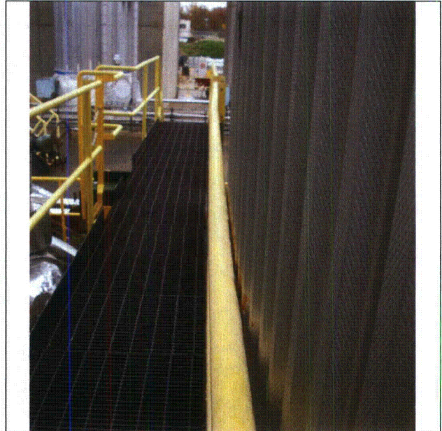
Note: Very small gap between platform and Primary Water Storage Tank.
