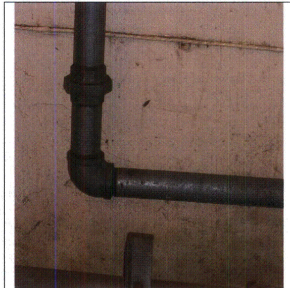
Note: Threaded pipe for the 26 sump pump discharge.
