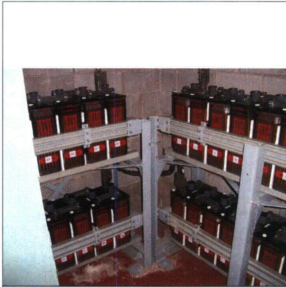
Note: Batter rack 23.
