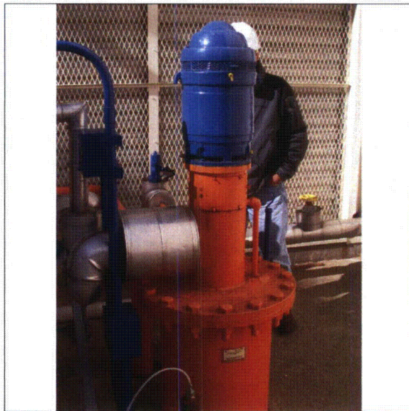
Note: Fuel Oil Transfer Pump
