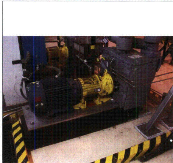
Note: View of pump
