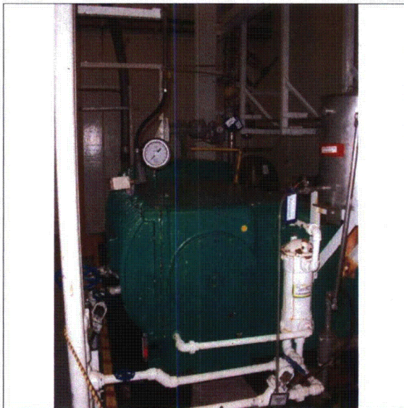
Note: View of pump
