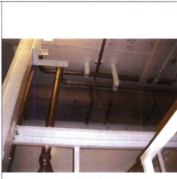
Note: Ductwork above pump
