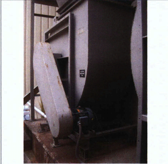
Note: Front view of the Exhaust fan 21ETEF
