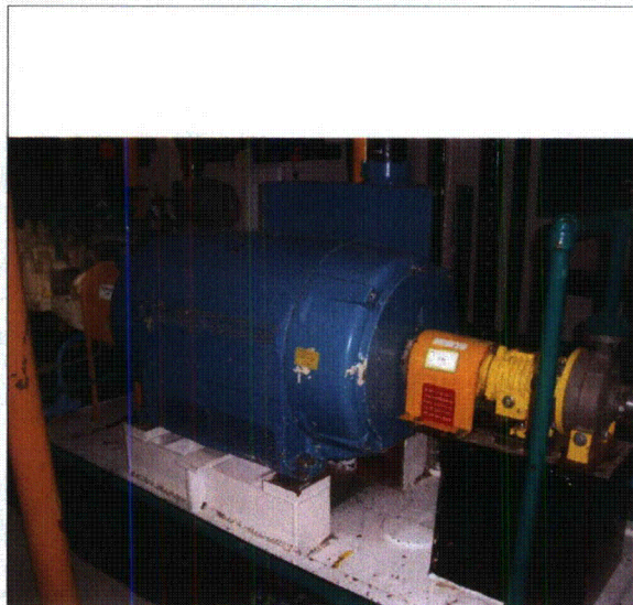
Note: The motor of the safety injection pump
