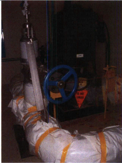
Note: Front view of the pump no 21
