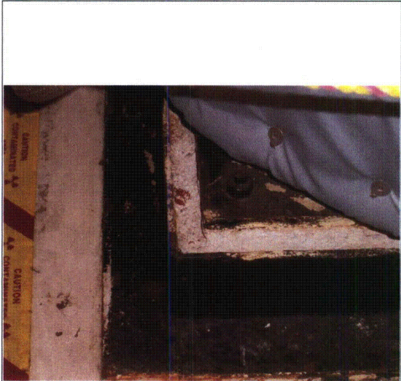
Note: Anchor Bolt view of the pump
