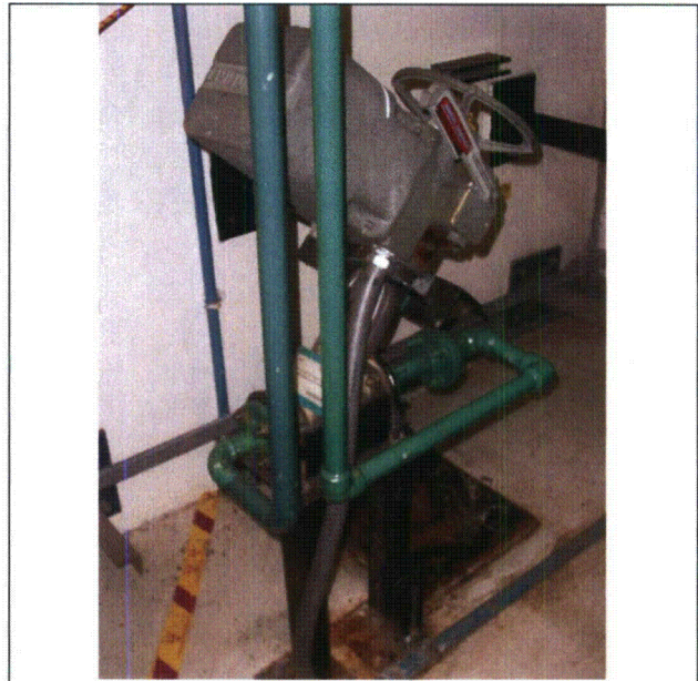
Note: Corrosion on the plate
