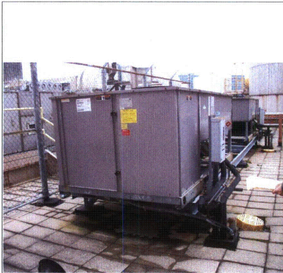
Note: The condensing unit, CCRAC2, with anchorage area covered with water proof materials
