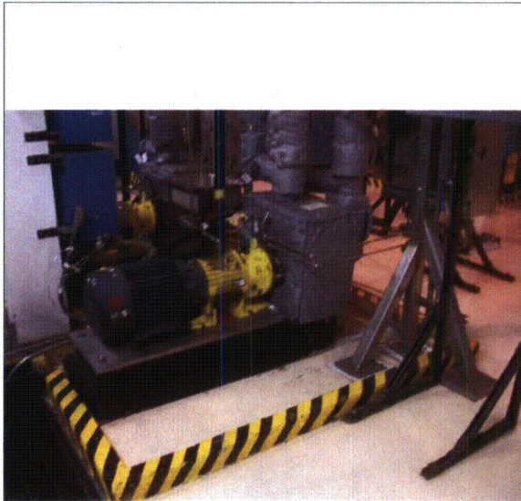
Note: View of pump
