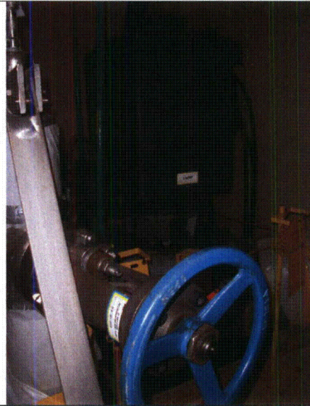
Note: Corner view of the pump
