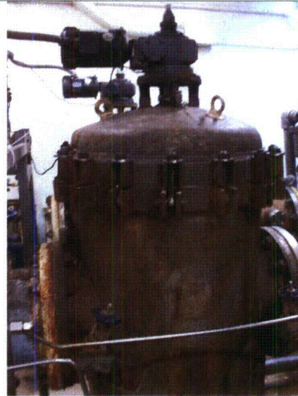
Note: Side view of the service water pump automatic strainer
