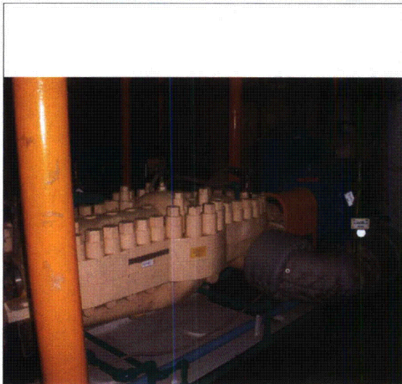
Note: 21 Safety injection pump, front view
