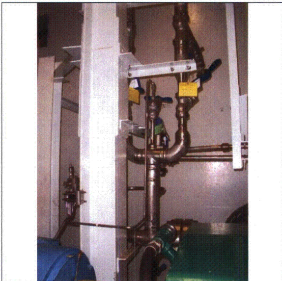
Note: View of piping in room
