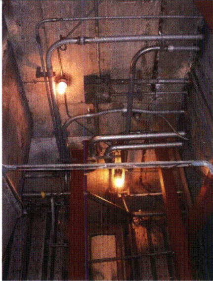
Note: Area, Above the fan 21
