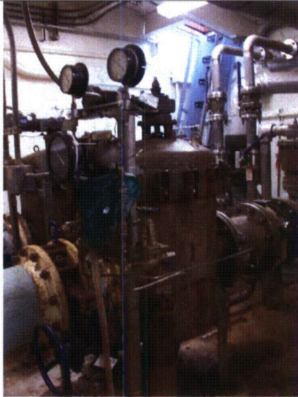
Note: Front view of the service water pump automatic strainer.
