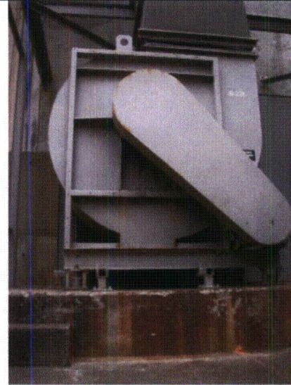
Note: Side view of the exhaust fan
