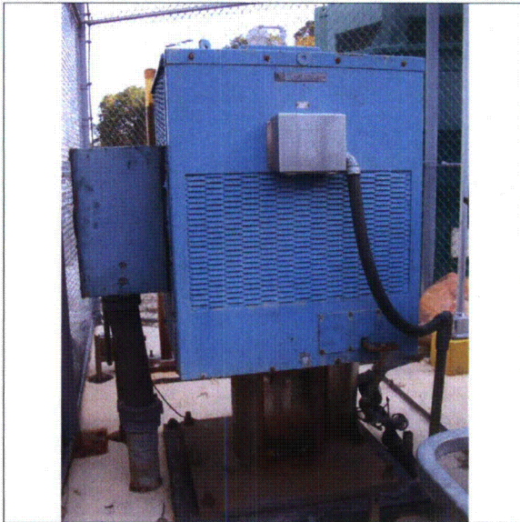
Note: 26 Service Water Pump
