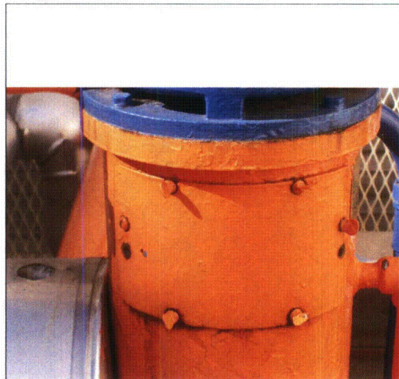
Note: Cover plate missing 2 of 8 screws.
