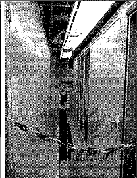
Note: Row of cabinets in Room 96.
