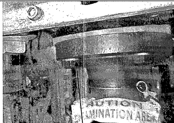
Crack in washer
