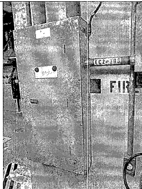
Note: General view showing the panel mounted flush against the wall.
