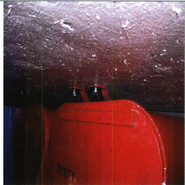
Note: Picture of the non-tightened/loose anchorage of the clean/dirty rag bins.
