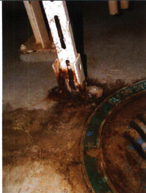
Note: Picture of the degraded anchorage of the UNISTRUT support.
