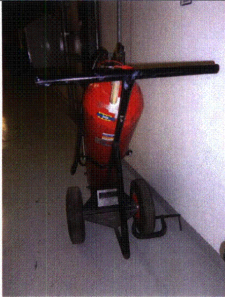
Note: CO 2 fire extinguisher 76CX-606
