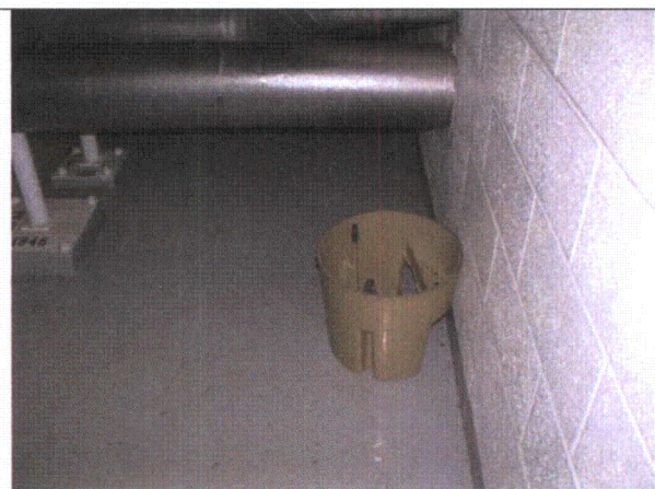
Note: Picture of a step ladder not in designated location in Pump Rom B.
