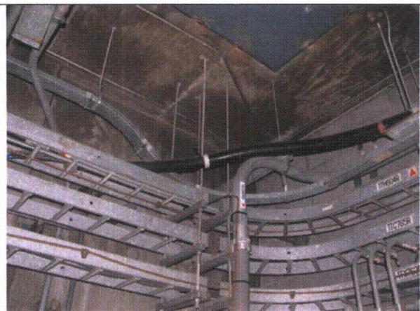
Note: Picture of the conduit tied to a rod hanger support the on cable tray 1TH604R1.
