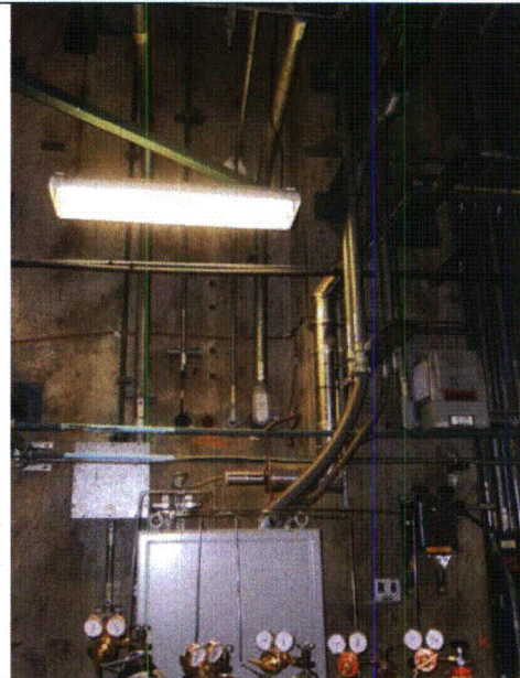
Note: Light fixture above 1/4" tubing from the gas tanks
