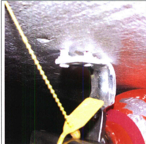
Note: PICTURE of the non-tightened/loose anchorage of the 76CX-609 hand held fire extinguisher.
