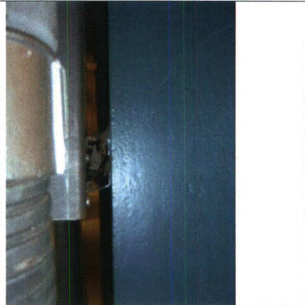
Note: Failed Unistrut Channel Nut, Refer to question 2.
