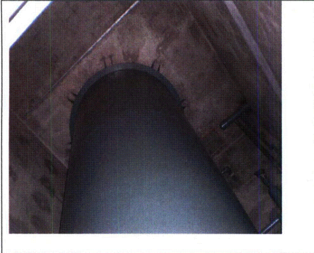
Note: 19TK-8A with anchorage at ceiling.
