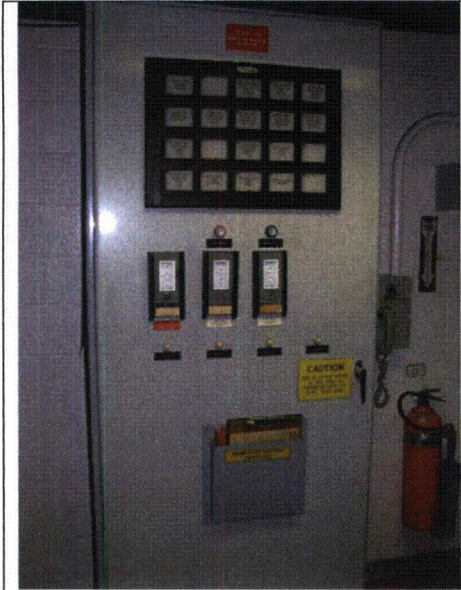
Note: Picture of equipment 72HV-7A.
