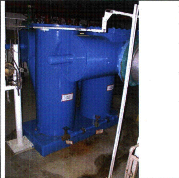
Note: Picture of equipment 46STR-5A2.
