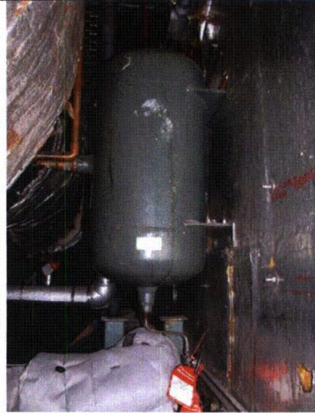
Note: Picture of equipment 29AC-1A.
