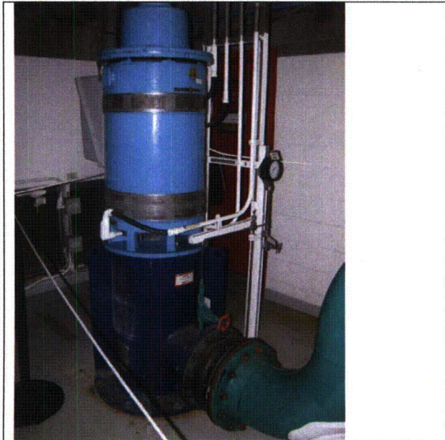
Note: Picture of equipment 46P-2A.
