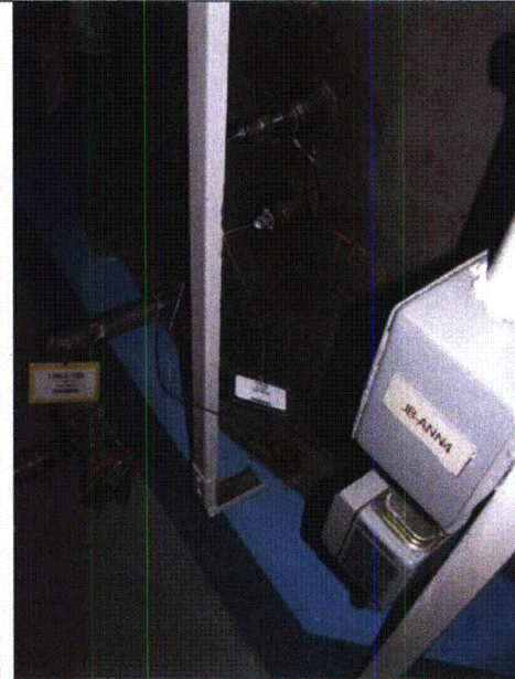
Note: Picture showing the element sensor wire (equipment 11TE-49) near the unsupported Unistrut support.
