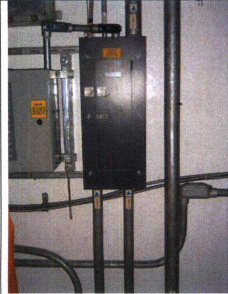
Note: 71ACB4 Distribution Panel
