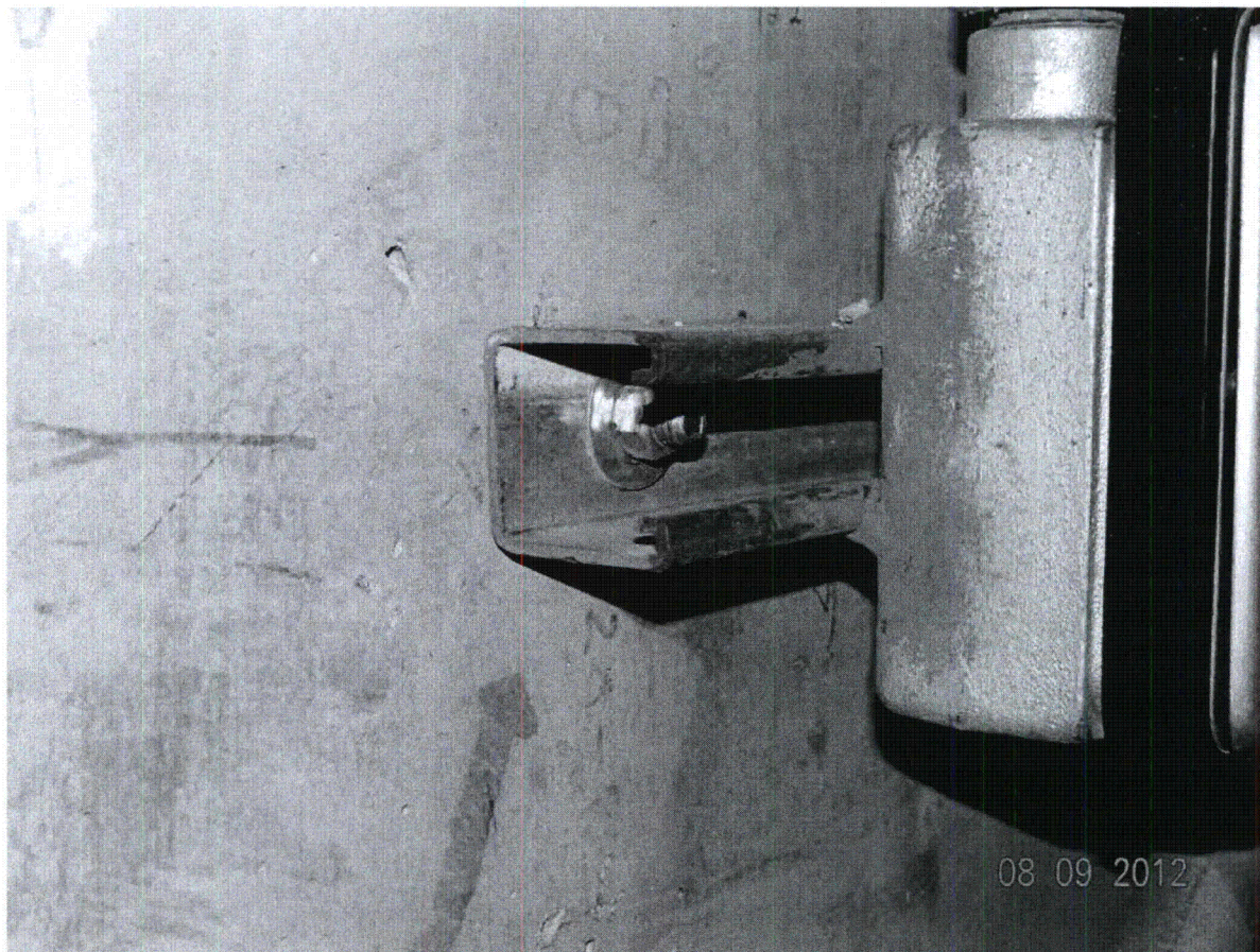
Picture DSC00342 "Bolt Configuration"
