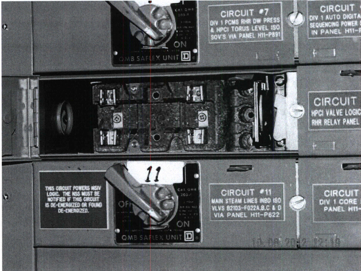
Photo 2, Close-Up View of Fused Disconnect Switch
