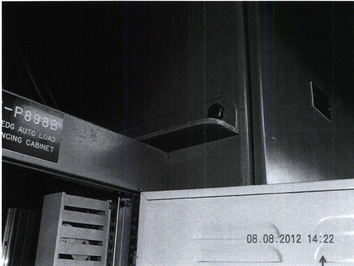
Seismic Bracing Bolt Configuration (Right Rear of Cabinet)
