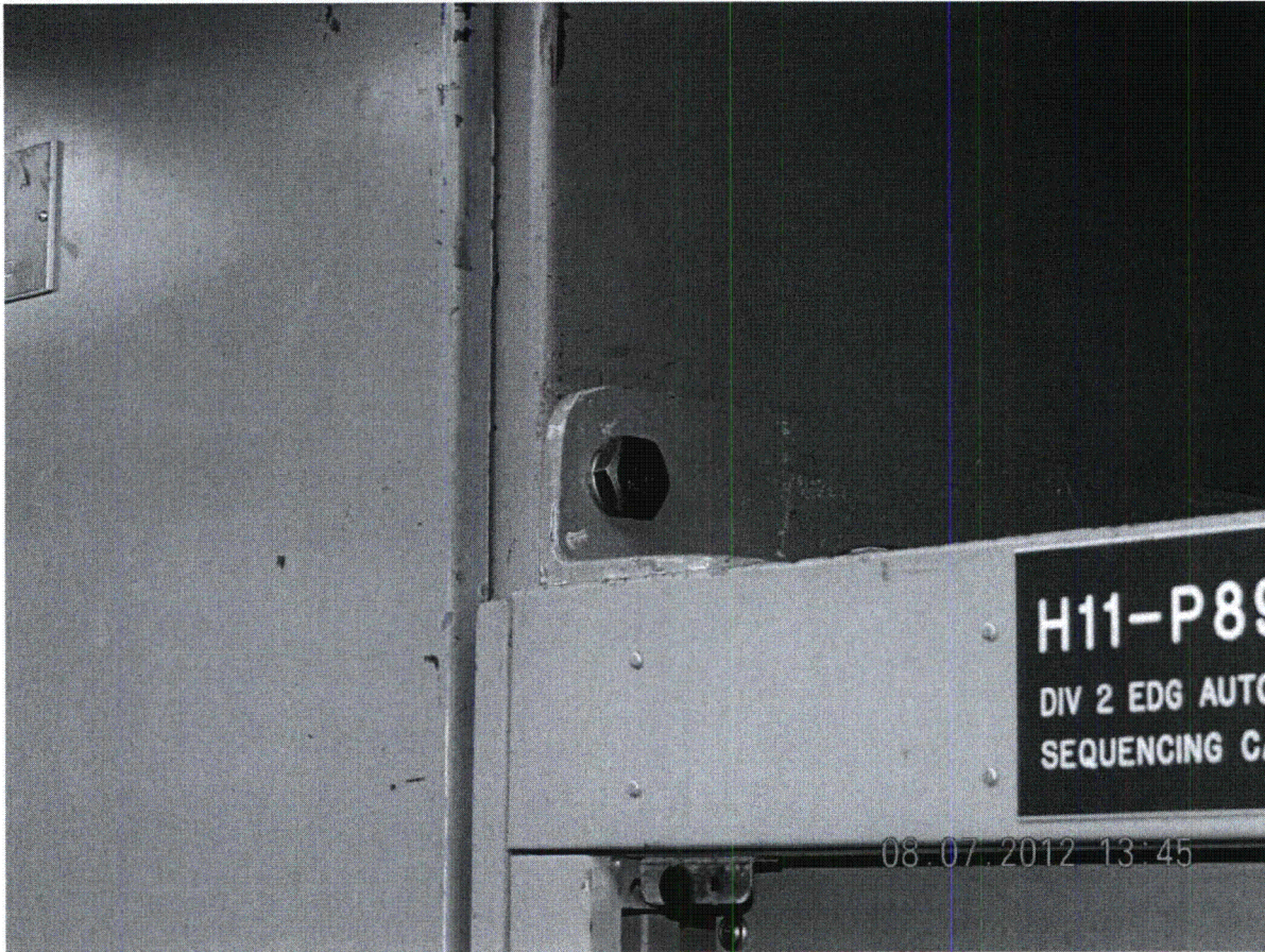
Seismic Bracing Bolt Configuration (Left Rear of Cabinet)
