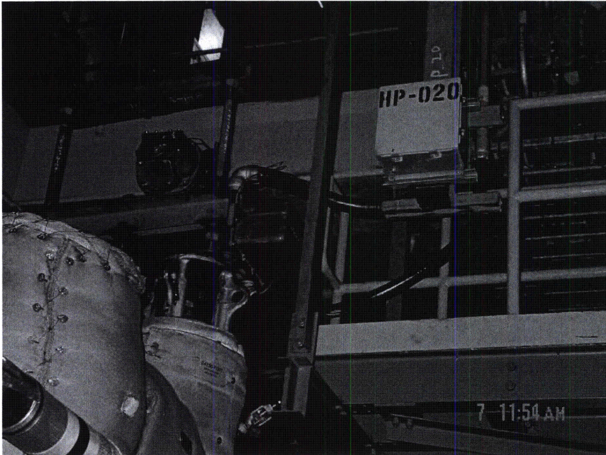
Flexible Conduit Lines to Motor Operator (Picture 5)
