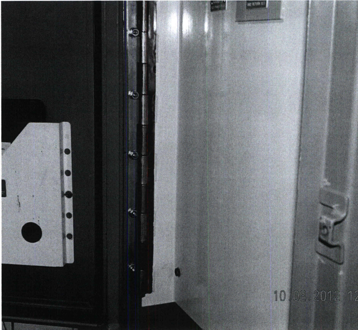
Photo 2, Close-Up View of Hinge on Left Side of Mounting Plate
