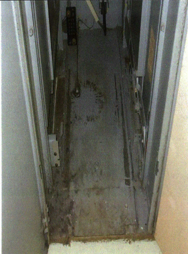
1AP06E Byron - de-energized Equip 9-22-12 008
