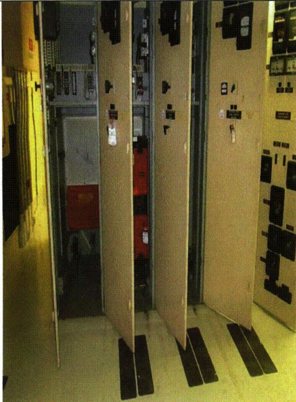
1AP06E Byron - de-energized Equip 9-22-12 007
