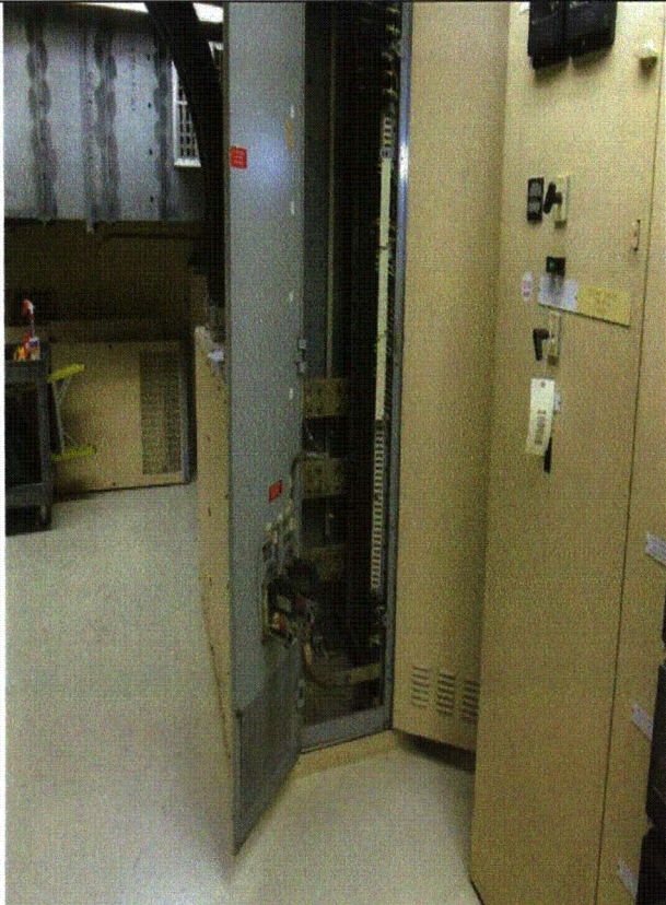
1AP12E Byron - de-energized Equip 9-22-12 016
