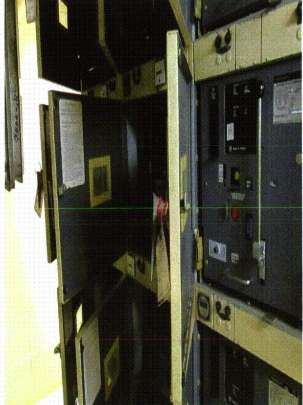
1AP12E Byron - de-energized Equip 9-22-12 019
