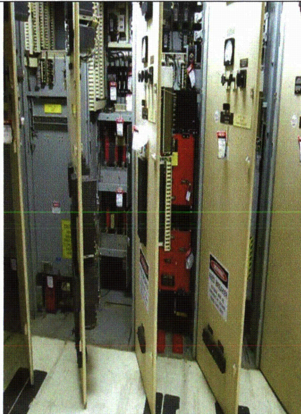
1AP06E Byron - de-energized Equip 9-22-12 006
