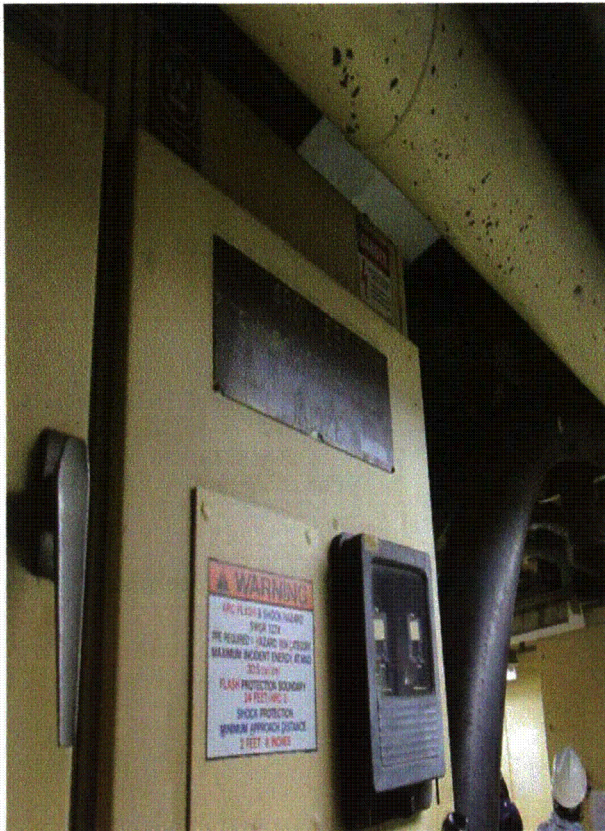
1AP12E Byron - de-energized Equip 9-22-12 011
