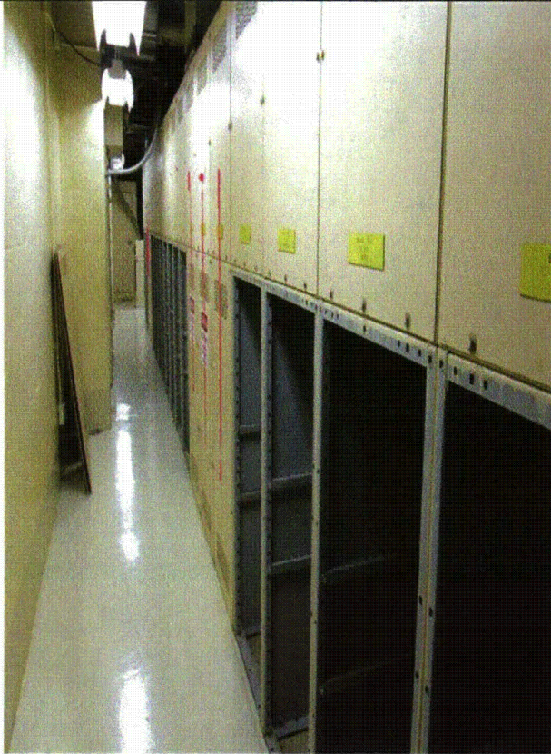
1AP06E Byron - de-energized Equip 9-22-12 021
