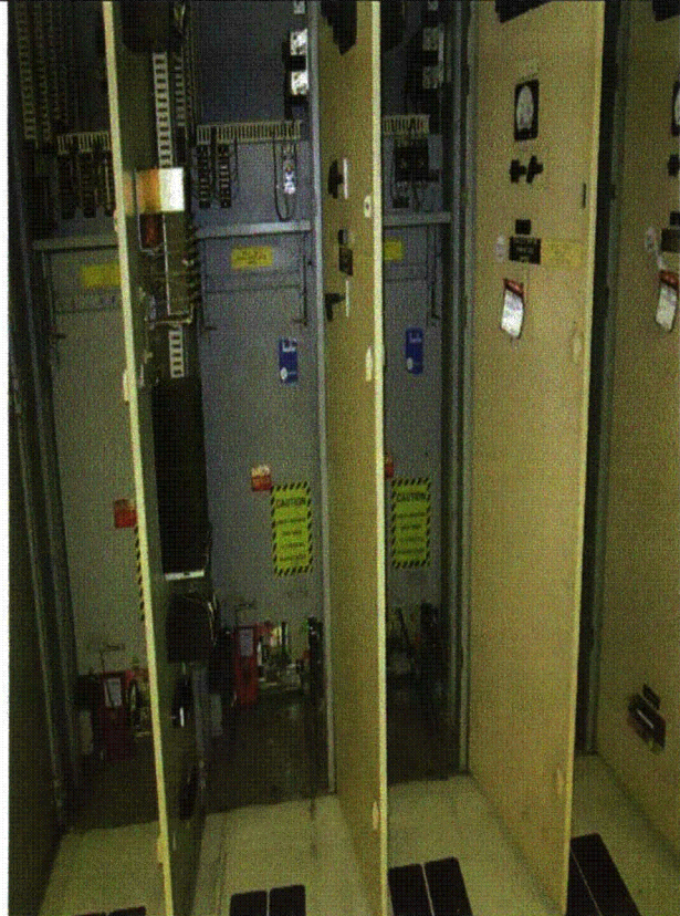
1AP06E Byron - de-energized Equip 9-22-12 004
