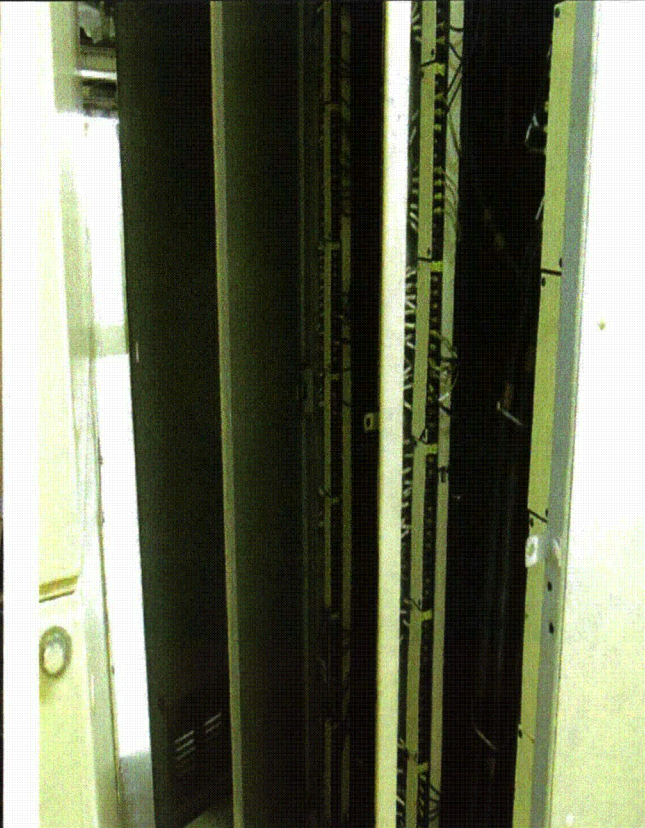
1AP12E Byron - de-energized Equip 9-22-12 017
