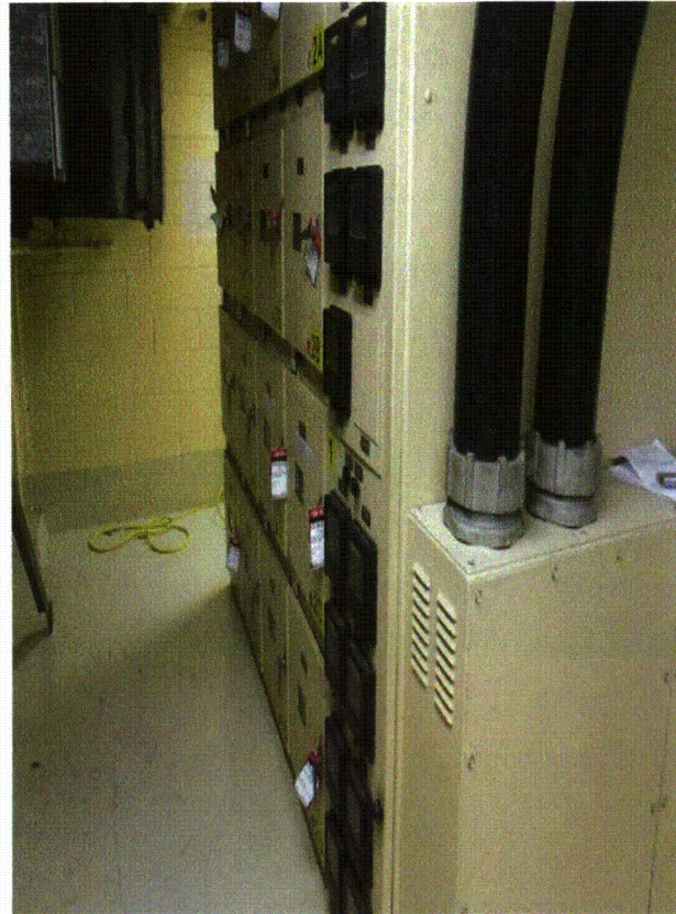
1AP12E Byron - de-energized Equip 9-22-12 013
