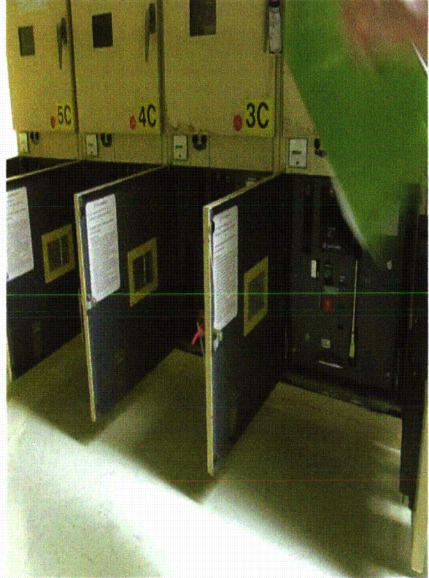
1AP12E Byron - de-energized Equip 9-22-12 015
