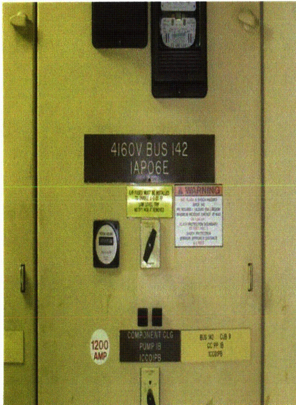
1AP06E Byron - de-energized Equip 9-22-12 001
