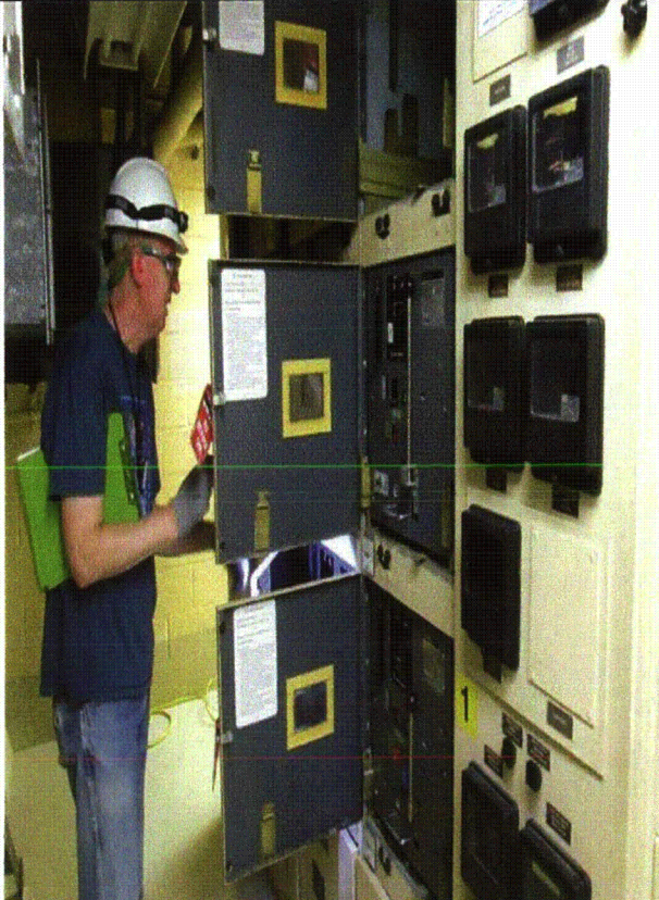
1AP12E Byron - de-energized Equip 9-22-12 018
