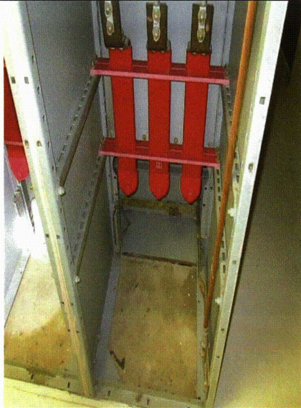
1AP06E Byron - de-energized Equip 9-22-12 022
