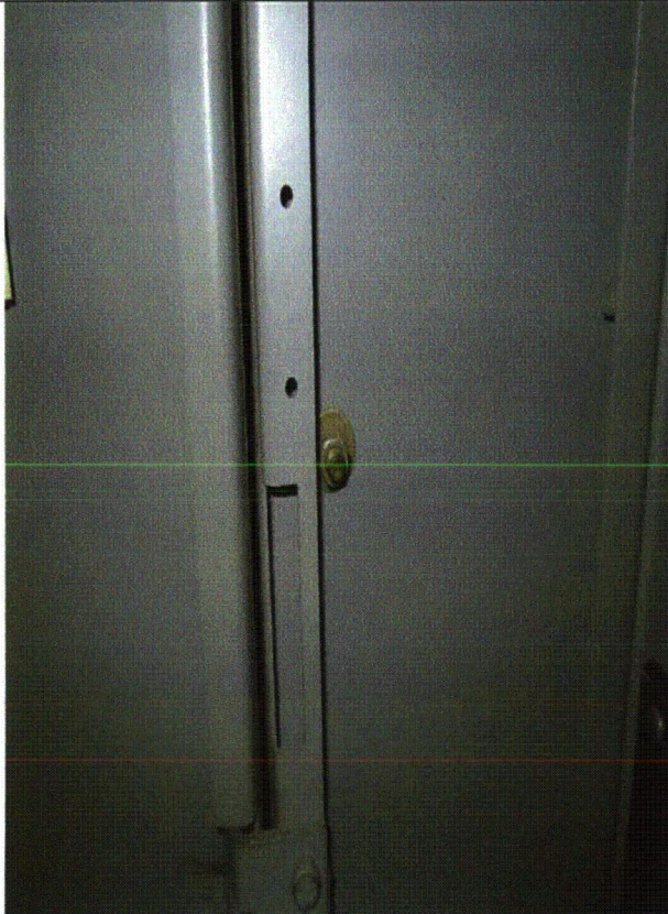
1AP06E Byron - de-energized Equip 9-22-12 009
