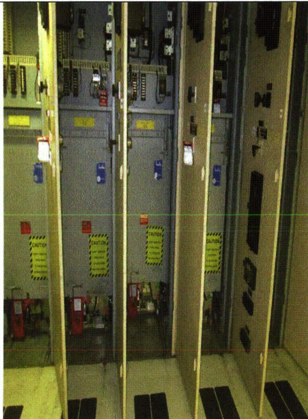
1AP06E Byron - de-energized Equip 9-22-12 005
