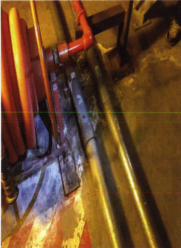
0VC09Y (NP-6695 WATER LEAK )Byron 1 & 2 041
