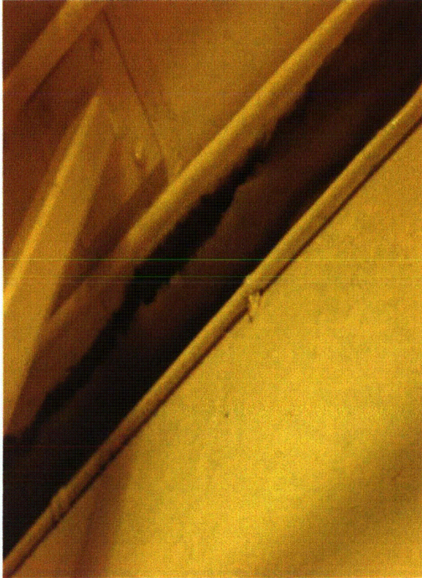
2MS001C (AWB - DAMAGED ISOLATION JOINT AND WEATHER STRIP) 8-1-12 AM 008
