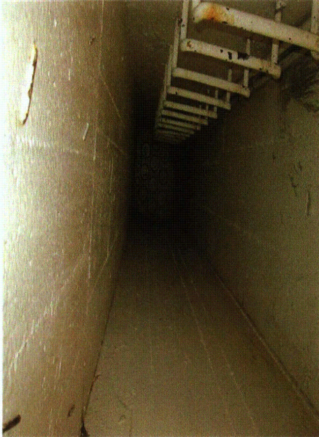
1LT-0932 (AWB - water leak from hatch) 7-19-12 017
