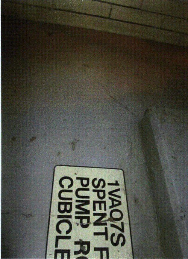
1FC01P (6695 - cracked concrete) 7-18-12 077
