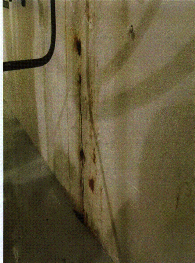
1CC01PB (AWB degraded concrete) 7-18-12 020
