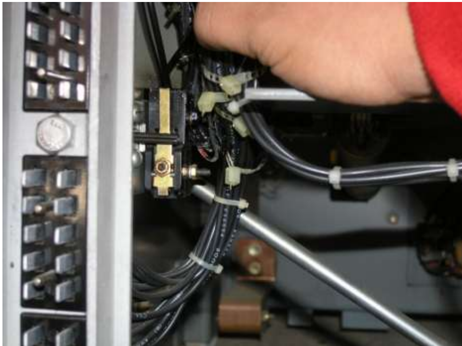
Figure A-46 Another view of damage to the wires located in the wireway between the connector block and the auxiliary contacts
