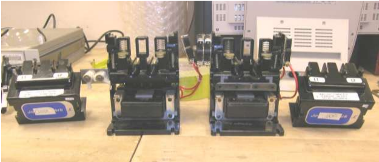
Figure A-8 Side-by-side comparison of the open and closed motor contactors for the MOV-2 circuit
