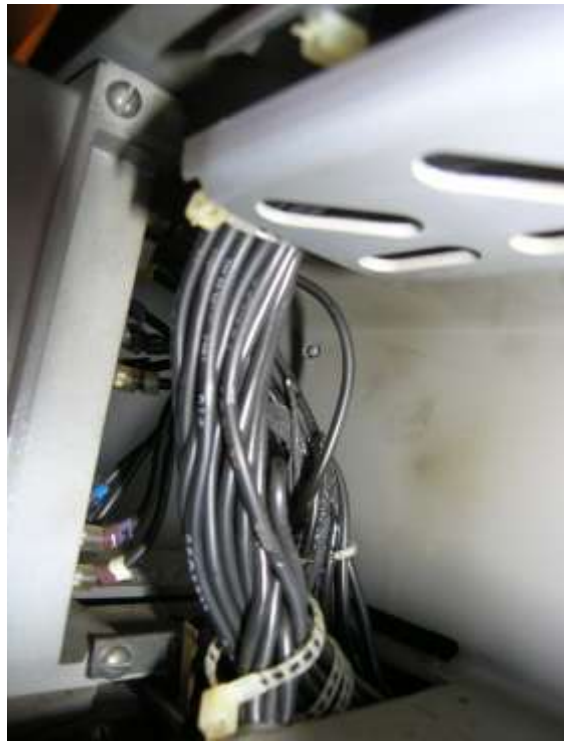
Figure A-44 Damage to some of the wires inside the bundle behind the connector block
