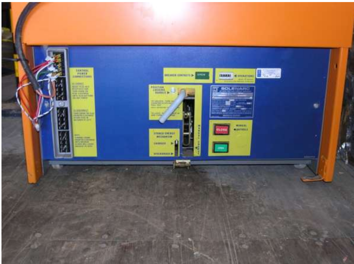
Figure A-41 Front of the switchgear unit. The return cable connections are being made at the left side.
