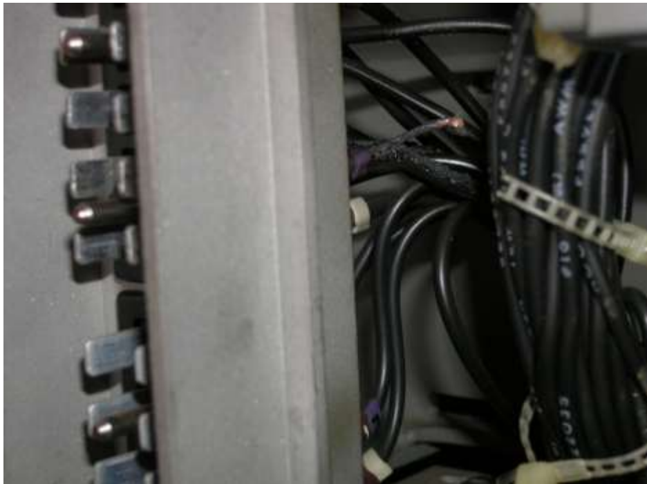
Figure A-42 Damaged panel wires immediately behind the connector block
