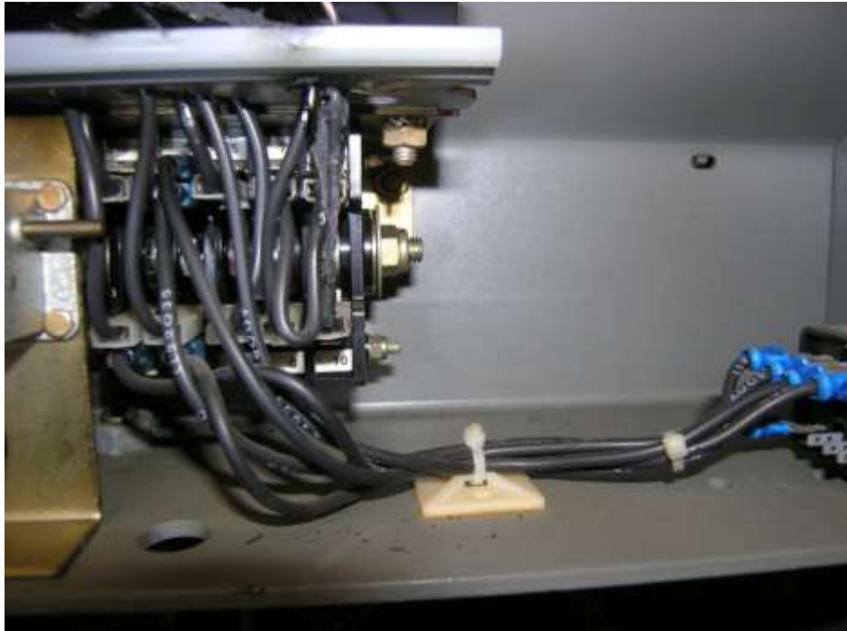
Figure A-48 Panel wire damage at the auxiliary contacts
