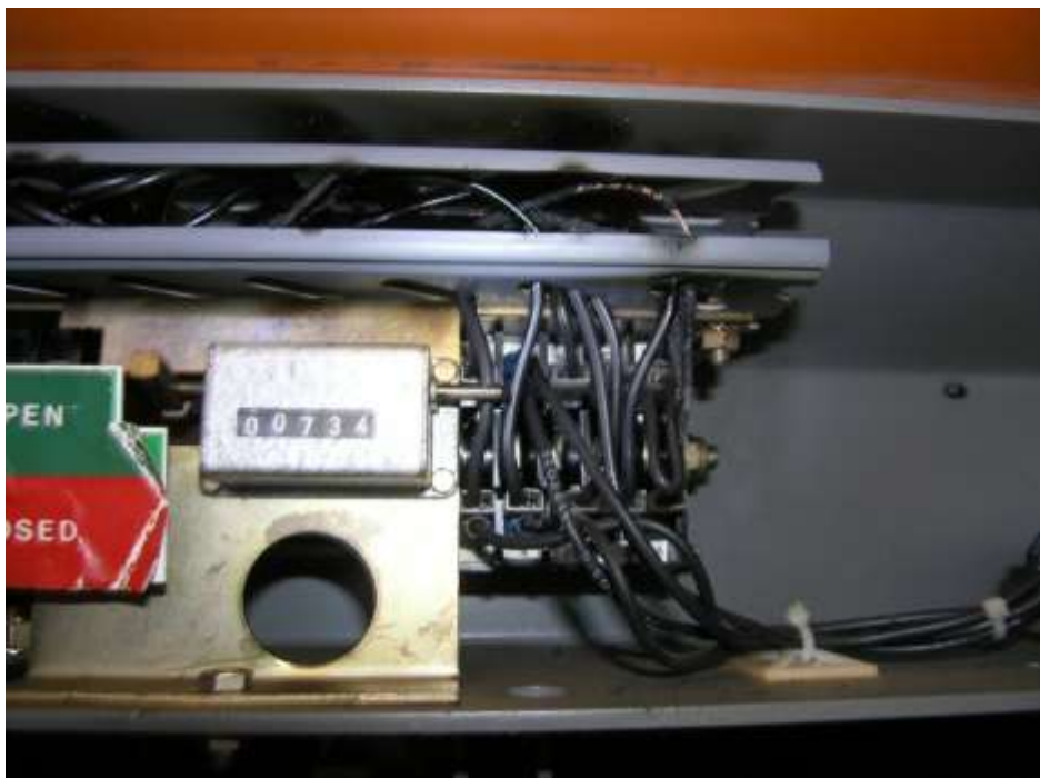
Figure A-47 Panel wire damage near the auxiliary contacts
