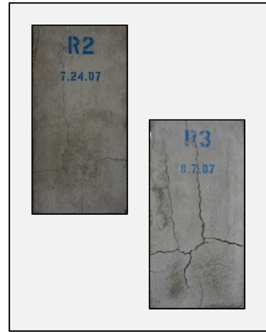
Current and Future Damage
