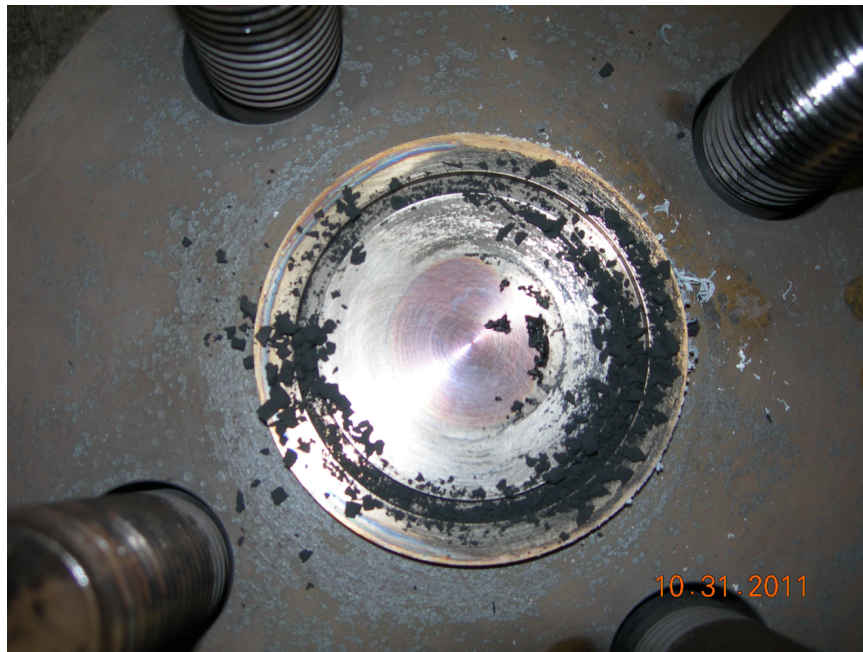
Figure 3-40. Photograph showing the disintegration of the tested ethylene-propylene compound O-ring when an attempt was made to remove the O-ring from the groove.
