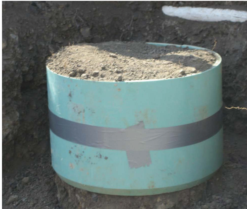
Fig. 3.4. Block sample being collected at ACAP test facility in Underwood, ND. Upper photograph shows sample partially trimmed into ring. Lower photograph shows sample in ring and ready for separation from subgrade.
