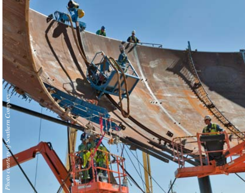
Above, welding on some of the 58 steel plates that will form the Vogtle Unit 3 containment vessel bottom head.
