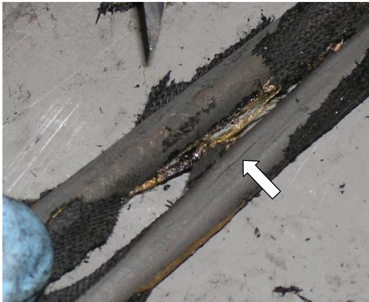
Figure 7.38: Longitudinal cracking observed during the post-test analysis is visible as a dark line running along the right hand conductor near the center of the photo.
