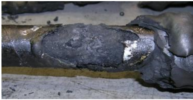
Figure 7.45: Close-up image of the large hole formed in the zinc wrap.
