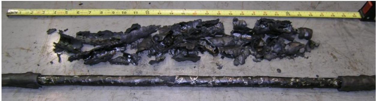
Figure 7.46: Jacketing material removed from the thermally exposed portion of the energized cable.
