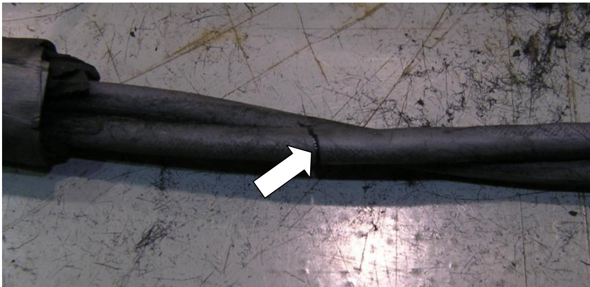
Figure 7.3: Circumferential cracking extending to the bare wire of Item A.
