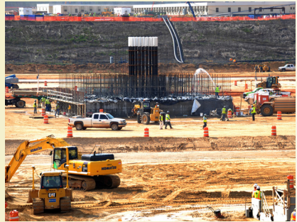
Preconstruction activity on limited work authorized at the Vogtle new reactor site.
