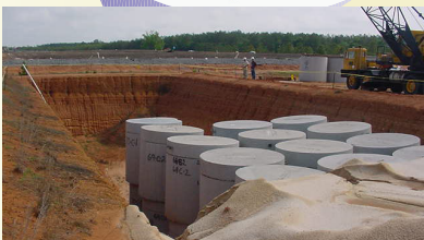
This LLW disposal site accepts waste from the compact States.
