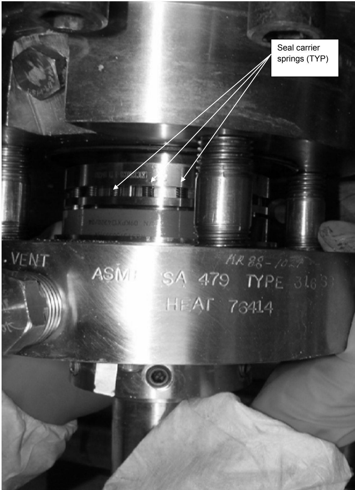
HPSI mechanical seal being disassembled
