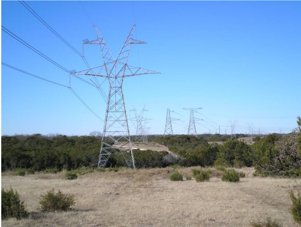
Figure 3-5. Oncor Transmission Line Towers with Vacant Circuit Positions (NRC Staff Photograph)
