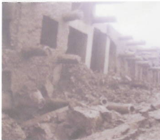
Pilings that were supposed to assure that the building was stable.
