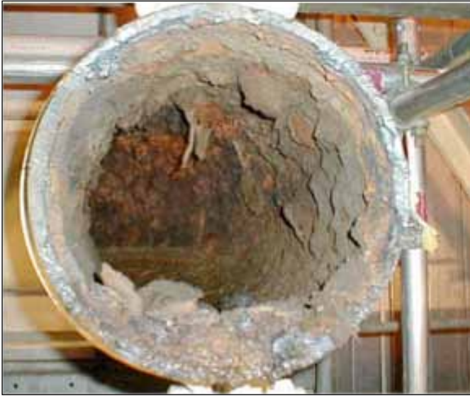
Figure 9.26 Corrosion and biofouling of carbon steel service water system piping
