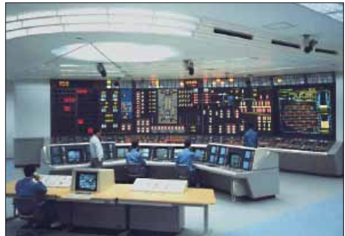
Figure 10.1 Highly integrated control room
