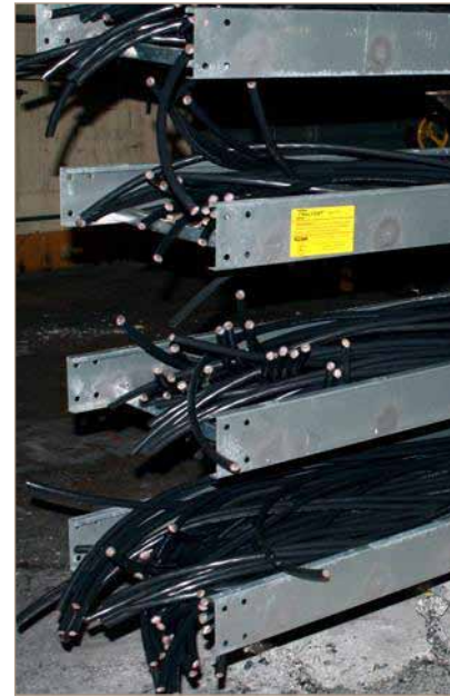
Figure 7.11 Cables in tray (Cables placed in trays before fire test)
