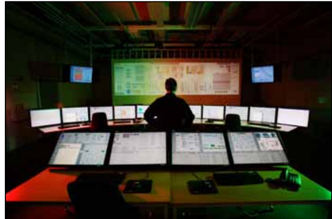
Figure 12.2 HAMMLAB control room simulator
