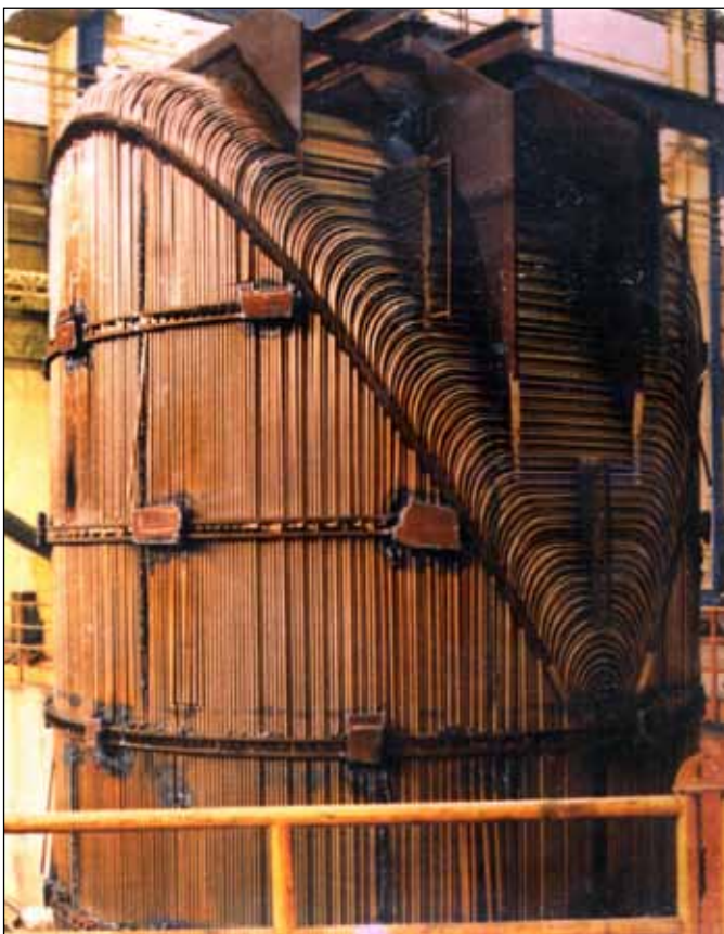
Figure 9.4 Recirculating steam generator tube bundle
