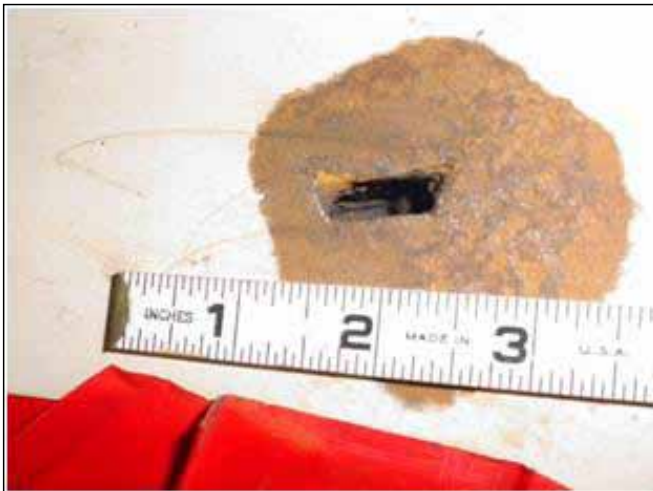
Figure 9.21 Photograph of the through-wall corrosion detected at Beaver Valley, 2009. A piece of wood embedded in the concrete during original construction was found behind the corroded area of the steel containment liner. The area was identified by a large paint blister which was filled with steel corrosion products.
