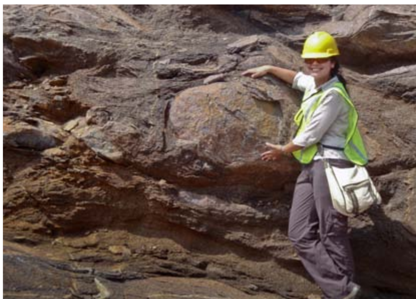
Right, NRO Geologist Meralis Plaza-Toledo examines rocks at the V.C. Summer Unit 2 excavation site in Fairfield County, SC.
